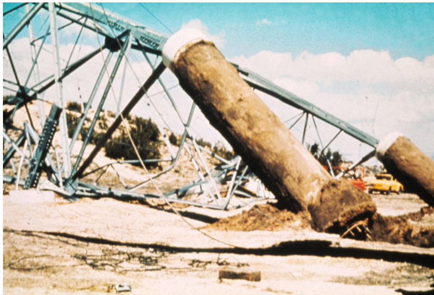
Figure 1.18 Failure of a 500 kV suspension tower drilled shaft foundation.
