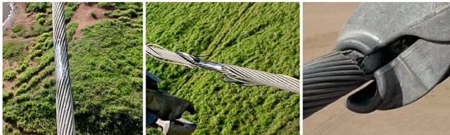
Figure 1.10 Wear and failure of conductor strands due to spacer clamp loosening.
