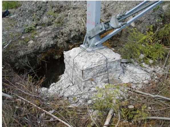
Figure 13.34 Separate foundations incorrect concrete mix design and curing (Key 8).
