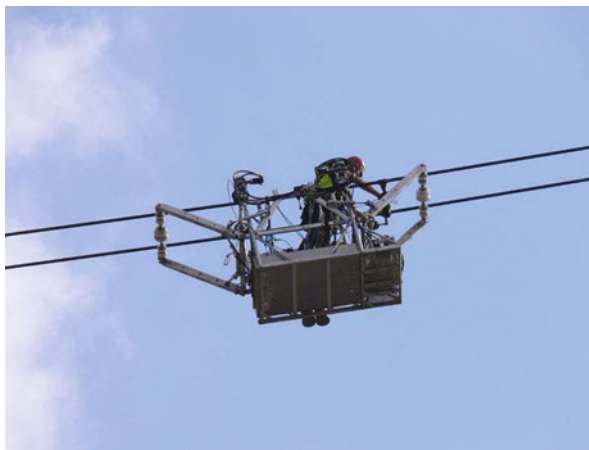
Figure 1.22 Cart used on a horizontal twin bundle.
