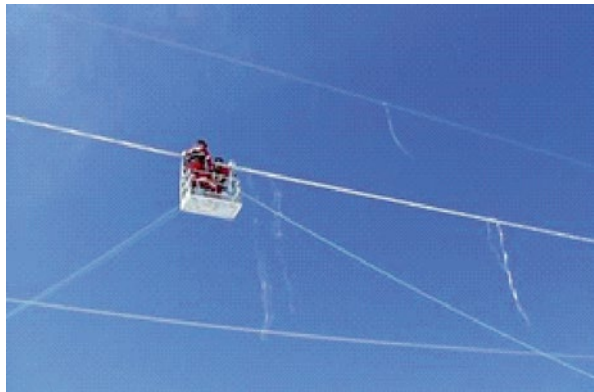
Figure 9.130 Repair of damage caused by shield wire clashing with conductors (ice shedding, galloping).
