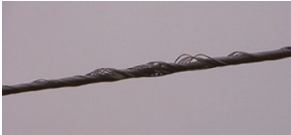
Figure 9.125 Birdcaging due to mishandling during stringing.
