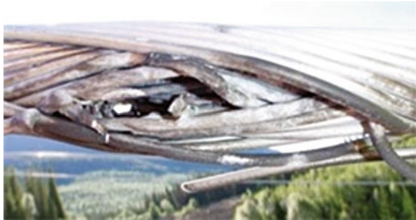
Figure 9.124 Lightning damage on conductor (shield wire above).
