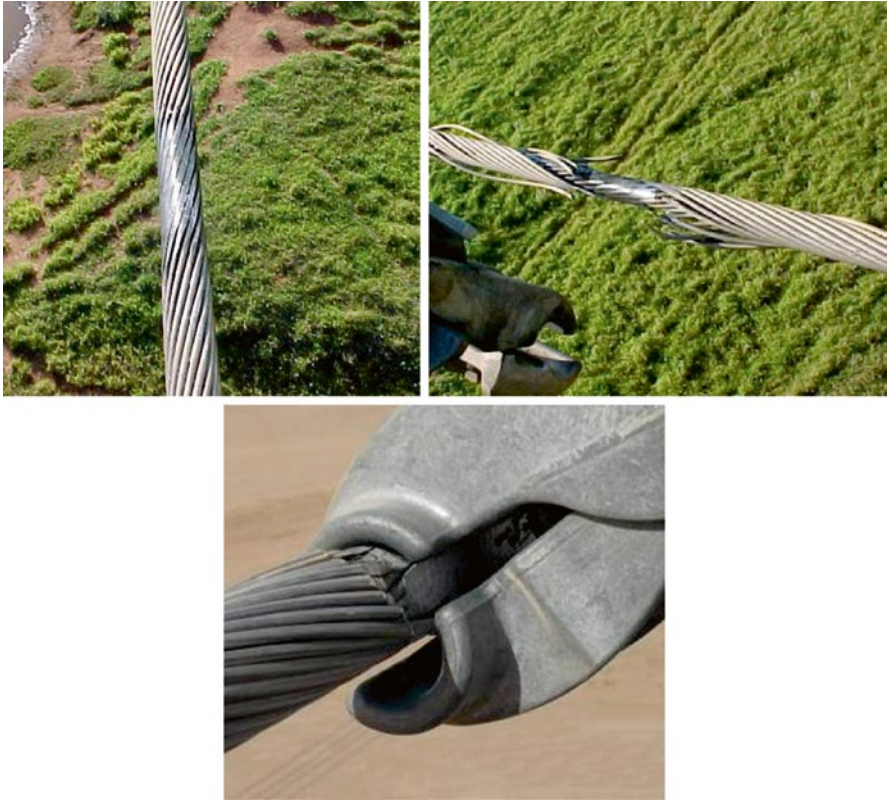
Figure 10.5 Wear and failure of conductor strands due to spacer clamp loosening.
