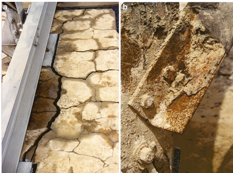
Figure 13.61 (a) Effect of AAR on concrete. (b) Steelwork corrosion.
