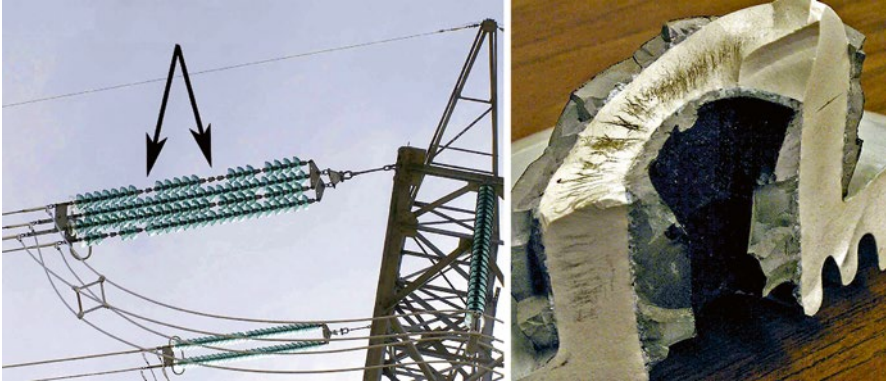
Figure 11.5 Broken shell of glass cap and pin insulators ( left ) and puncture paths inside a porcelain insulator cap ( right ) (Mishra et al. 2006).
