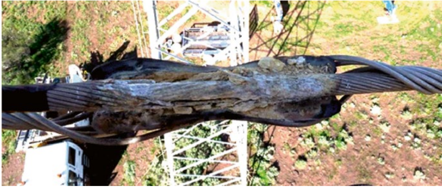
Figure 9.81 Corrosion damage inside elastomer-lined clamp caused by electrochemical incompatibility between the rubber and the conductor.
