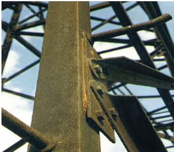
Figure 16.7 Corrosion at tower joints.
