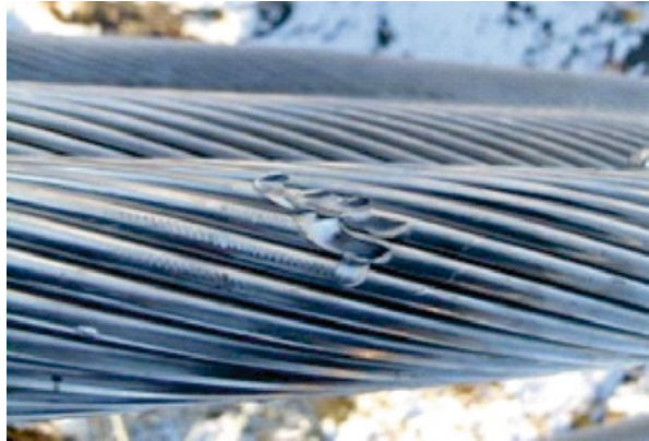
Figure 9.128 Aluminium damaged due to bicycle cart.
