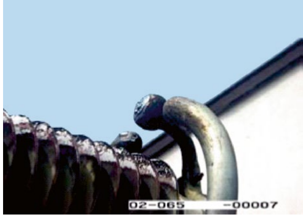
Figure 9.13 Arcing ring after 30 kA for 0.5 seconds.
