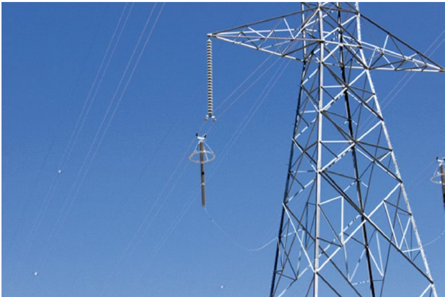
Figure 9.35 Surge arrester installed on twin bundle.
