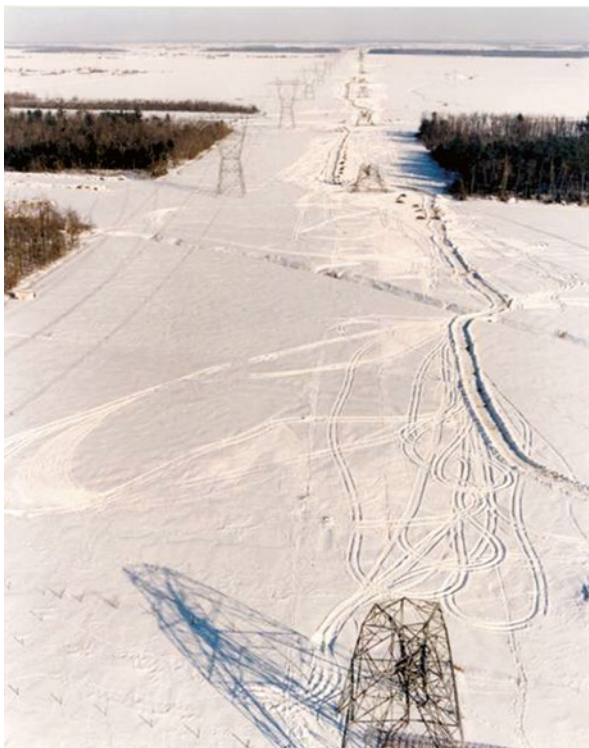
Figure 5.15 Longitudinal cascade on a 735 kV line in Canada during the Great Ice Storm of January 1998 (Photo: B. Breault, La Presse, Montréal ).
