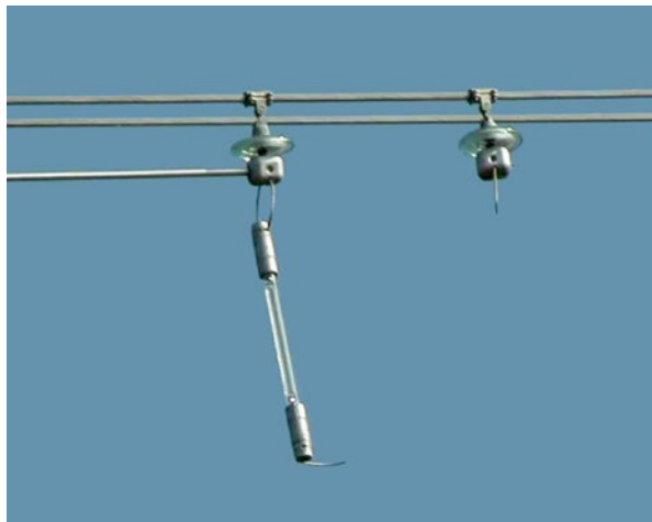
Figure 10.6 Night warning device, with a natural frequency around 20 Hz, broken by fatigue due to conductor vibration.
