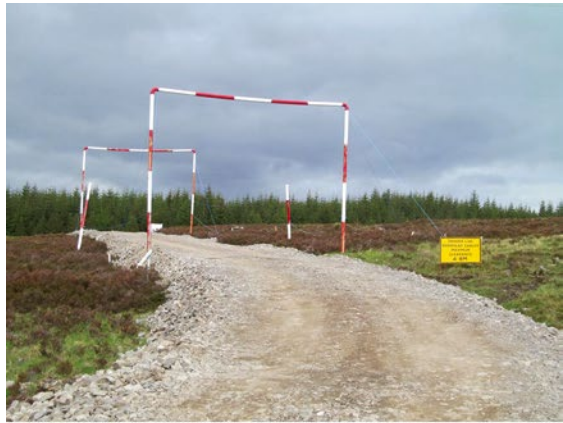
a) Temporary stone access road. Note use of height restriction 'goal post'
