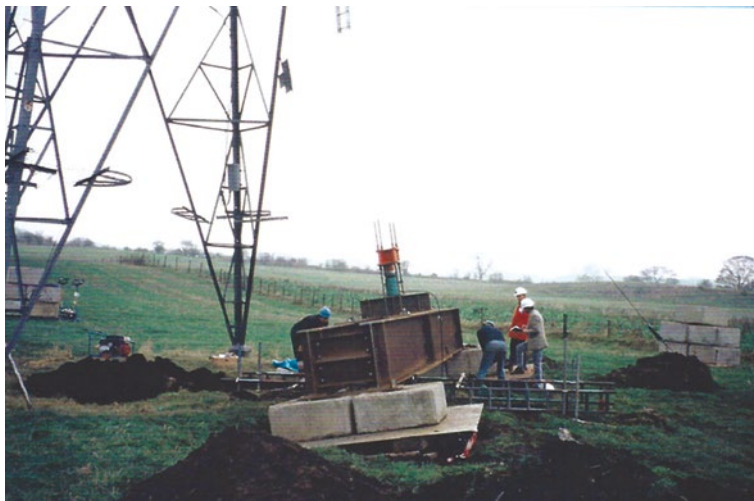
Figure 13.43 Full-scale testing of an existing foundation – support in-situ. (Note: Bottom tower leg disconnected and removed during the test)
