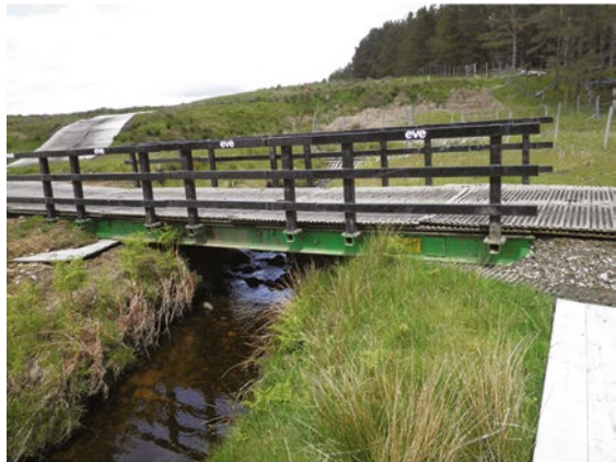
b) Temporary access track using aluminium track way panels and temporary bridging over a stream
