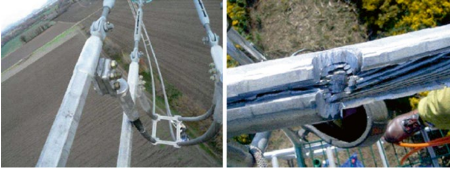
Figure 9.131 Damage to compression dead-end caused by clashing of jumper end fitting.
