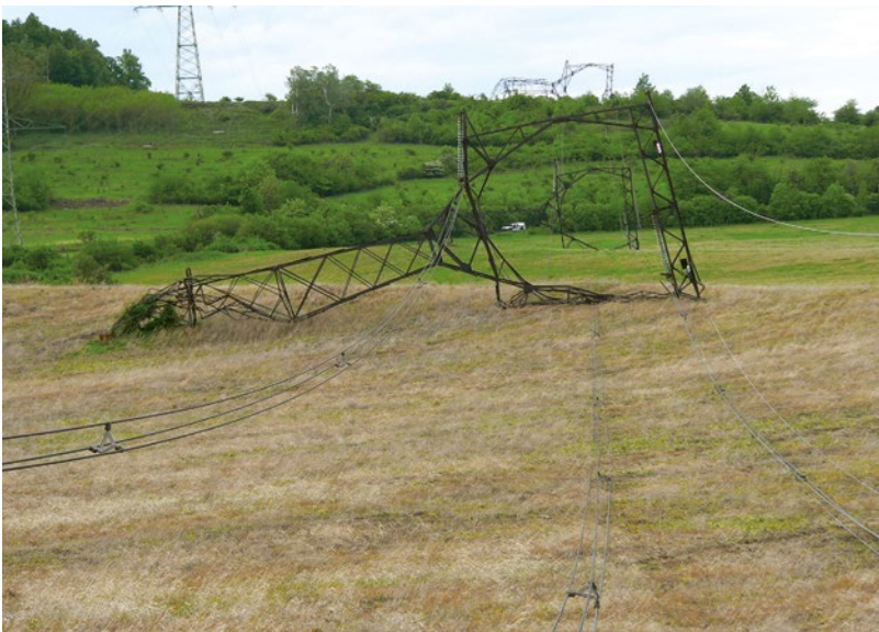
Figure 5.18 Transverse cascade of five 400-kV towers due to a May 2006 a High Intensity Wind (HIW) storm in Czech Republic (Photo: P. Froněk).
