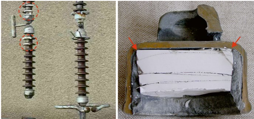
Figure 11.7 Power arc damage to porcelain longrod ( left ) (Cigré WG B2.21 2008) and cone breakage due to stress enhancement by non-rounded cone in the interface between porcelain and steel cap ( right ) (Cigré WG B2.03 2006).
