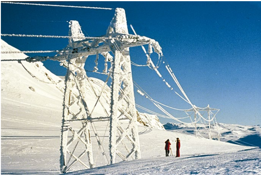
Figure 7.13 Rime icing on a 420 kV line in Norway, 1400 m above sea level (Photo: S.E. Hagen).
