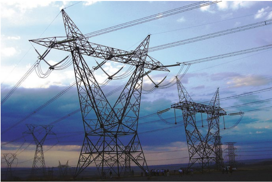
Figure 12.2 500 kV Anchorage Tower.
