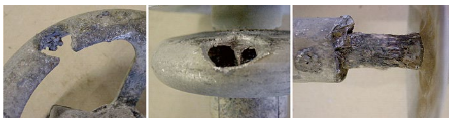
Figure 11.53 Power arc damage to an aluminium corona ring ( left ), aluminium corona collar ( middle ) and intensive thermal deterioration of the polymeric housing due to the aluminium combustion (Cigré WG B2.21 2008).
