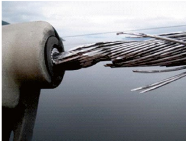
Figure 9.80 Wear and abrasion damage caused by a loose damper clamp resting against a warning marker clamp.
