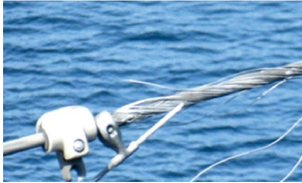
Figure 9.79 Wear and abrasion damage caused by a loose damper clamp resting against a warning marker clamp.
