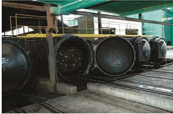
Figure 12.52 160'-long treating cylinders.
