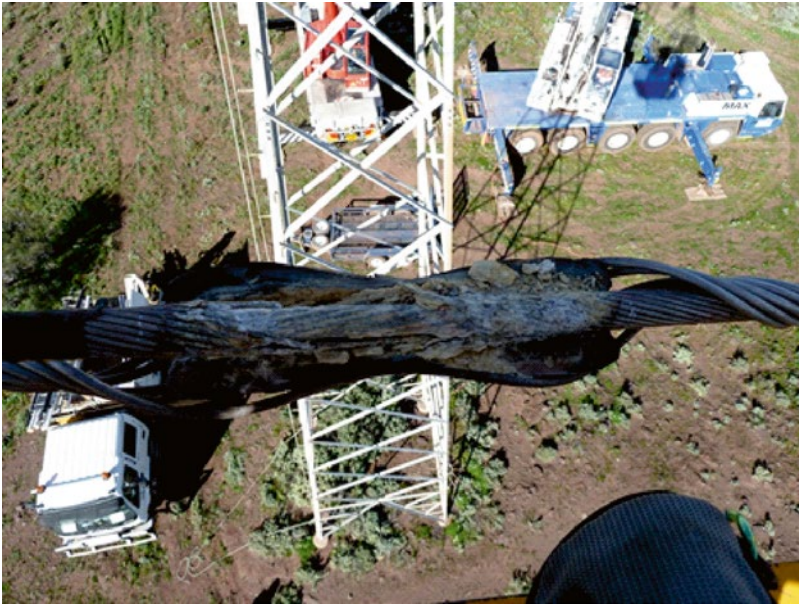
Figure 9.7 Corrosion inside a rubber cushioned clamp helically attached.
