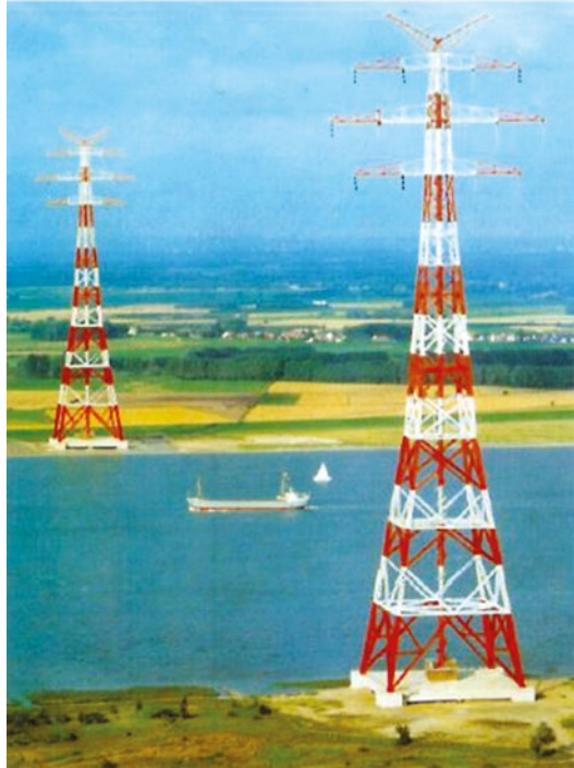
Figure 12.69 4 × 380 kV - Elbe River Crossing, Germany.
