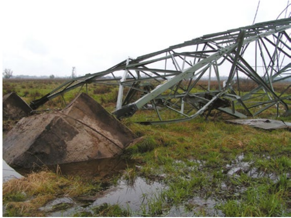
Figure 15.8 Foundation uplift. The right hand foundation is intact.
