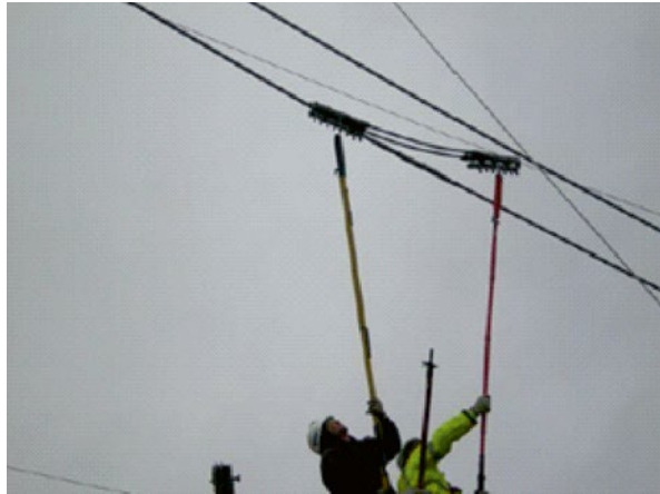
Figure 9.160 Installation of a bolted shunt on an energized line using hot sticks.
