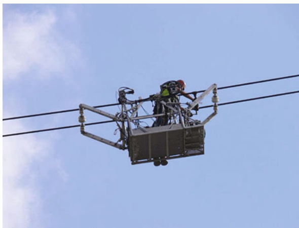
Figure 16.10 Cart used on a horizontal twin bundle.
