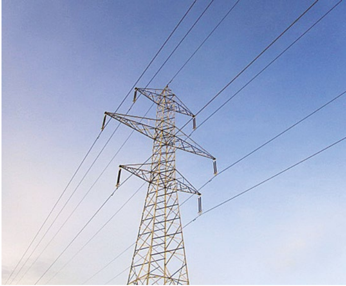
Figure 17.1 Typical 220 kV double circuit lattice steel tower.
