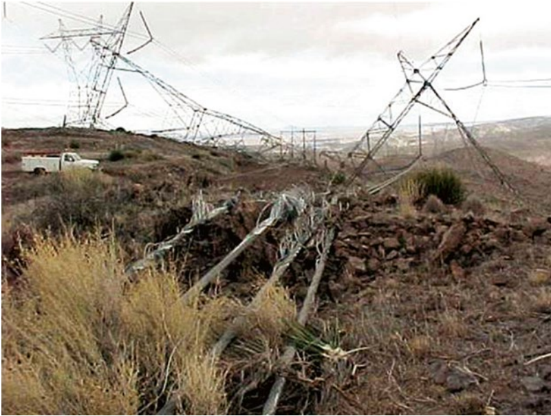
Figure 5.17 Transverse cascade on the 400 kV D/C Rubí-Vandellós-Pierola line in Spain during a 2008 a High Intensity Wind (HIW) storm (Photo: J. Santana López).
