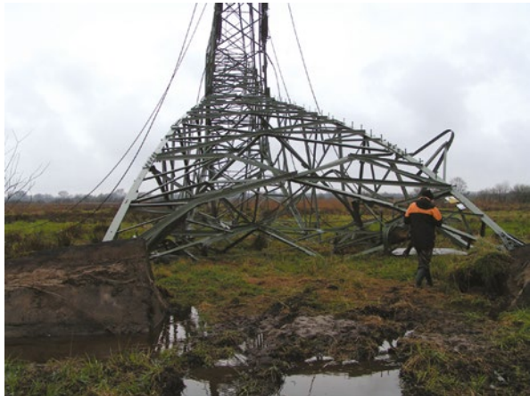
Figure 15.9 Destroyed tension tower of a 220 kV OHL.
