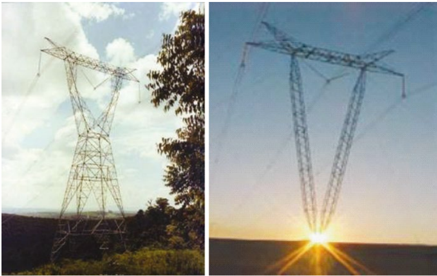
Figure 12.5 Self-Supported and Guyed towers.
