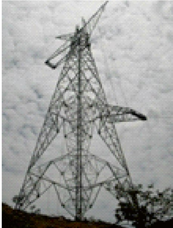
Figure 15.18 Section Method – a cross arm section of an angle tower is erected using a gin pole.
