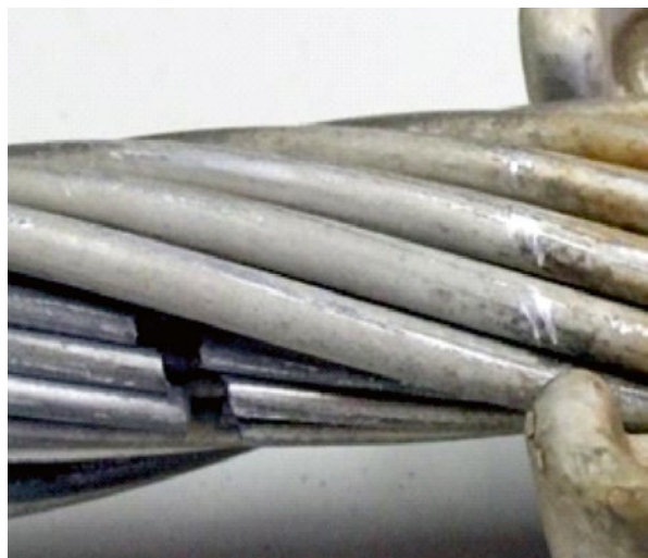
Figure 9.75 Fatigue failure underneath helical fittings.
