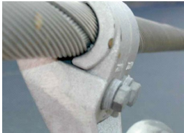
Figure 9.74 Fatigue failure at vibration damper clamp.
