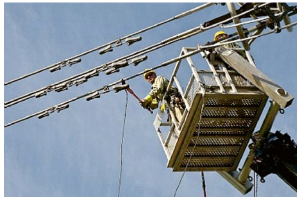
Figure 9.83 Stockbridge dampers on a quad bundle of a river crossing.
