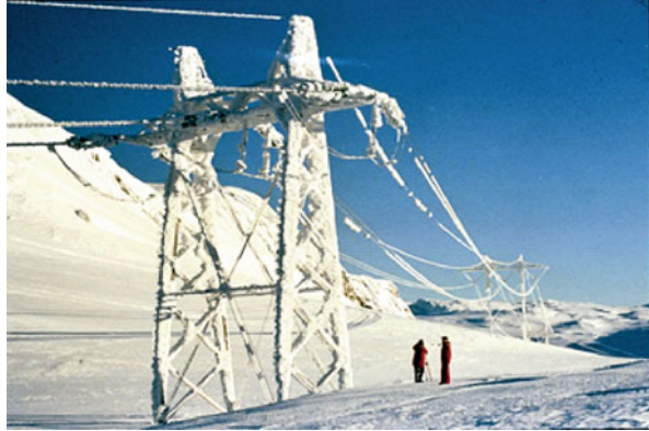
Figure 1.6 Rime icing on a 420 kV line in Norway, 1400 m above sea level.
