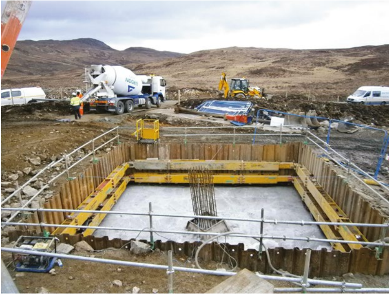
Figure 13.54 Intermediate stage concrete pad cast prior to placing stub and chimney formwork.
