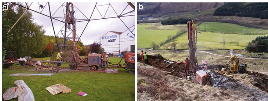
Figure 13.28 Combined cable percussion and rotary boring rig (a. existing tower, b. new tower site).
