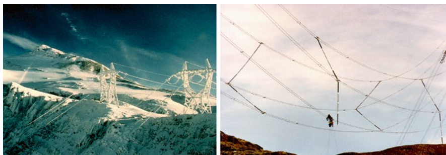
Figure 11.72 Winter situation at the highest European 420 kV line across the Alps ( left ) and introduction of interphase spacers to prevent conductor drop by ice shedding ( right ).
