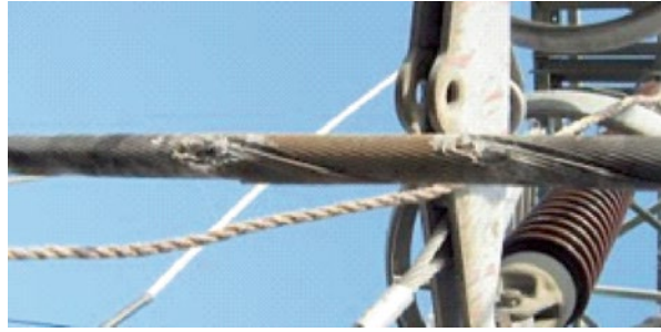
Figure 9.123 Lightning strike and flashover damage.
