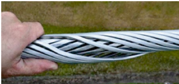
Figure 9.126 Birdcaging of ACSS/TW conductor.
