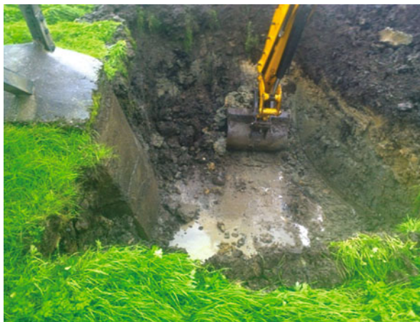
Figure 16.9 Foundation condition below ground.
