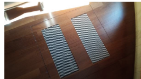
(e) Air duct on the floor
