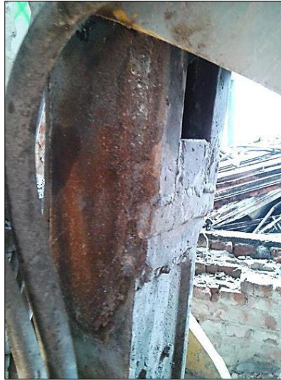
Fig. 2. Fatigue failure on the robot arm due to works in resonant frequency during the demolition process.
