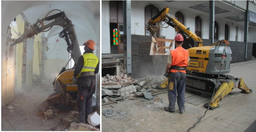
Fig. 1. Demolition robot and its operator with a remote control during various works (courtesy of ARCAD Ltd [12]).
