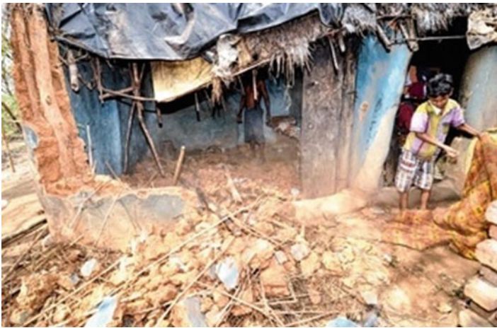
Plate 6.2 Hut damage due to elephant attack
