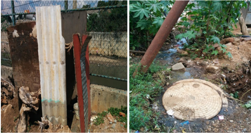
Photo Urban flooding adds to the menace of poor quality toilets and blockage causing leakage in manholes, Ventateshwara slum, Bengaluru
