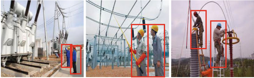
Fig. 1 Three images of transformer substation containing “person”. The red box indicates the location of person. A large variation of pose, appearance and scale is observed in these images
