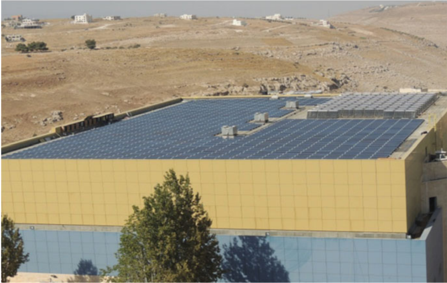
Fig. 61.2 PV plant on roof of cultural foundation forums building (ARENA) in AAU, Amman, Jordan
