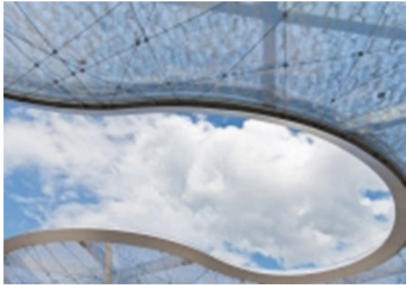
Fig. 3.5 Example of ETFE membrane; the airtight cushion offers shelter while allowing light to pass through its transparent form (photo by Niklaus Spoerri)
