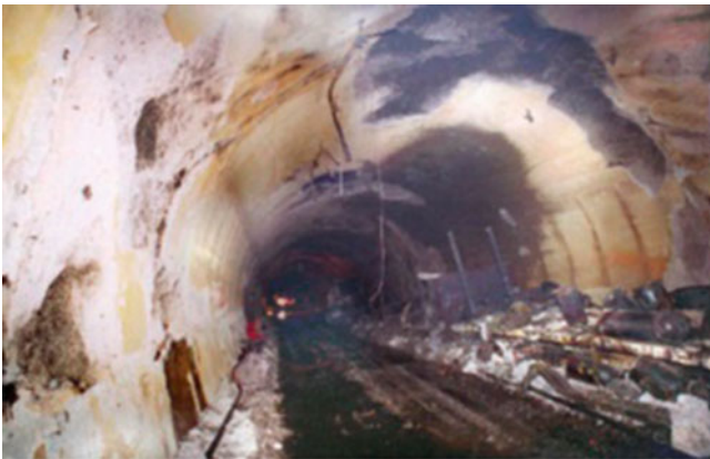
Fig. 1.9 Aftermath of the fierce fire that claimed 39 lives in the Mont Blanc tunnel (source http://www.tunneltalk.com )
