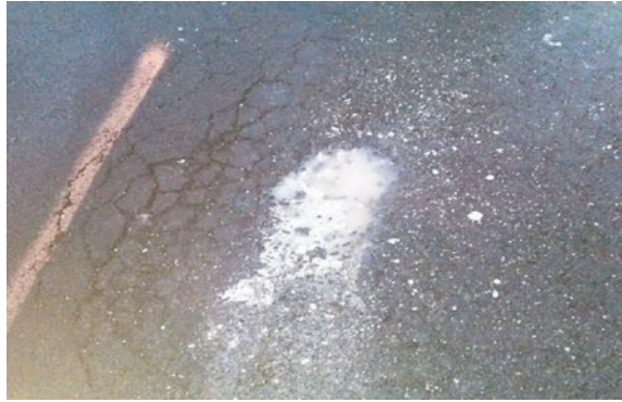
Fig. 3 Cracking and collapse of asphalt top seal laid down on 15/12/15 at Seaman's valley, Portland, Jamaica. Note cavitating soft limestone bedding, dissolution of calcium carbonate in acidic rain water, and cracks formed around it in the asphalt surface seal. Photo Herve Anderson 30/12/15. Source usgs.gov
