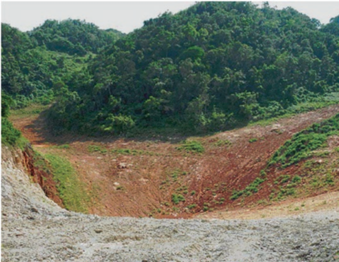
Fig. 1 A steep minesoil having a slope exceeding 15 % from the horizontal. Note the thin soil, suggesting a condition before capping, or, the erosion of applied capping. Source Jamaica Bauxite Institute
