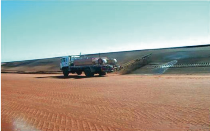
Fig. 9 Bitumen emulsion being sprayed to reduce dust from embankment walls. Adapted from Alcoa World Alumina Australia, March 07.
