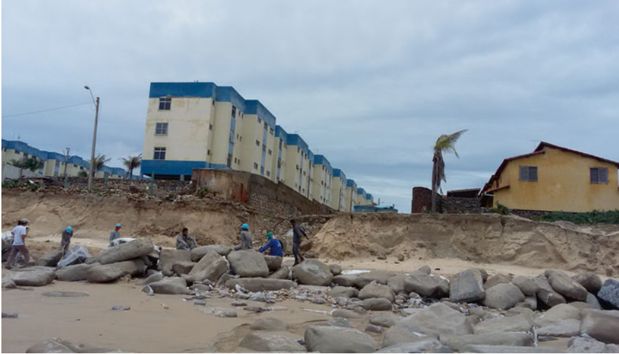
Fig. 7.14 Severe erosion at Icaraí beach hitting urbanization
