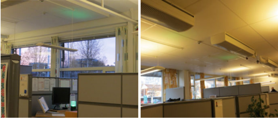
Fig. 6.6 The reflection of the “NEAT Lamp” on the ceiling represents an intersection between interaction design and architecture
