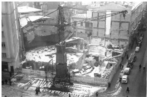
Fig. 18 Carlton building—the site and the crane in the final removal of debris. A part of cinema hall roof is still hanging, damaged (Pragher 1941)
