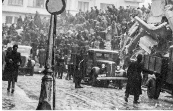
Fig. 12 Carlton building—the details of N–W wing collapsed balconies, on the right, seen from Regala Street (Galmeanu A (2015))
