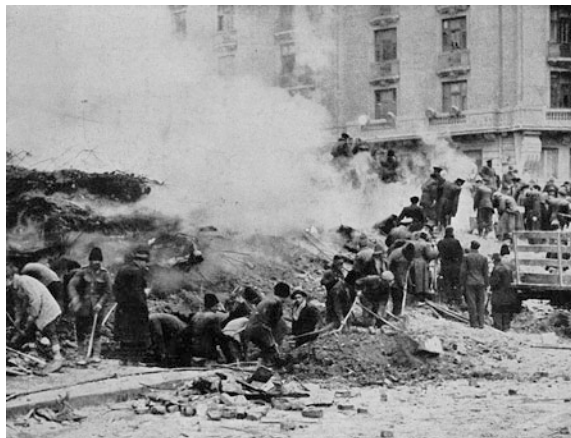
Fig. 16 Carlton building—digging by unskilled volunteers to reach the basement, while smoke is still present (L'Illustration 1940)
