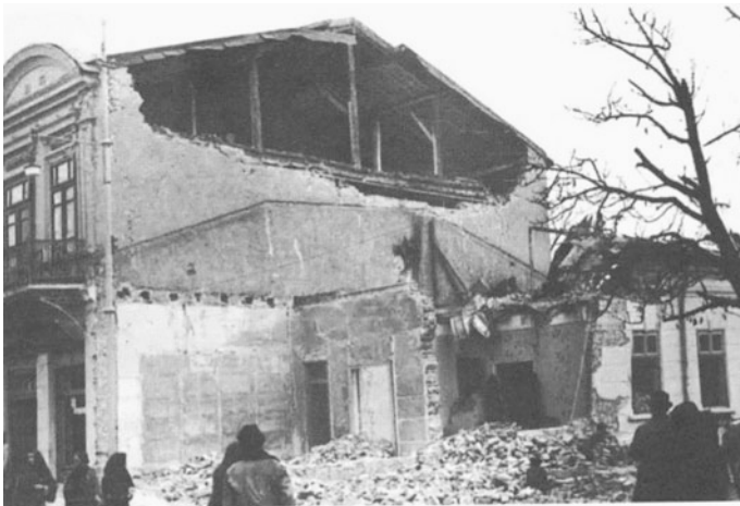
Fig. C.2 Fallen brick gable wall completely destroyed a next door smaller house in Focșani (Mândrescu 2008)
