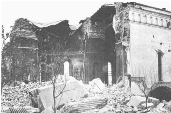
Fig. C.13 Close up view of the completely destroyed church in Crucea de Jos (Mândrescu 2008)
