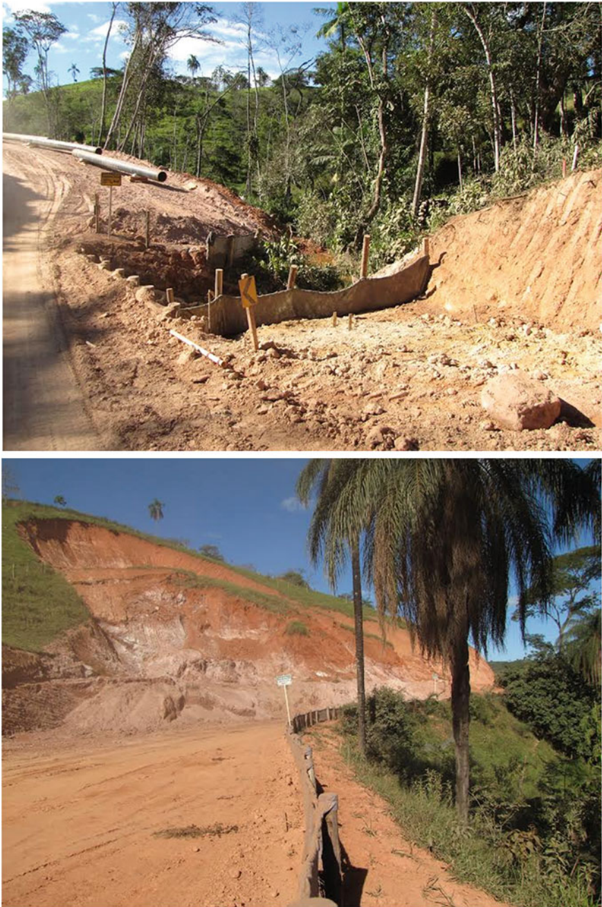
Fig. 21.8 The installations of the largest ore pipeline in the world in the region of Conceição do Mato Dentro (municipality of Santo Antônio do Rio Abaixo, Minas Gerais) caused many social and environmental damages. a Silting of springs and creeks in a rain forest and riverine vegetation; b large landslides with active erosions draining into springs and rivers. Photos G. Wilson Fernandes
