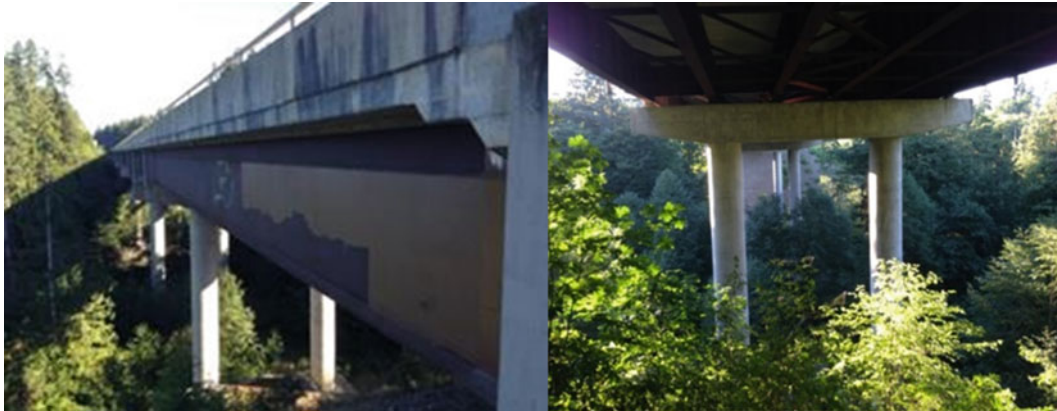
Fig. 19.2 Side view of concrete deck-steel girder system ( left ) and piers in middle spans ( right )
