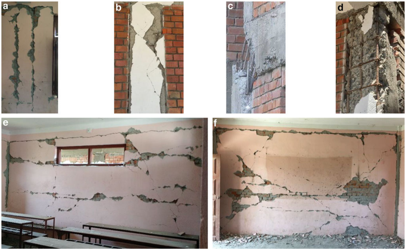
Fig. 5.4 Damages observed in the first-story of the school building at Sankhu during the earthquake. (a) Column G1, (b) Column G2, (c) Column H1, (d) Column H2, (e) Infill panel H12, (f) Infill panel E12
