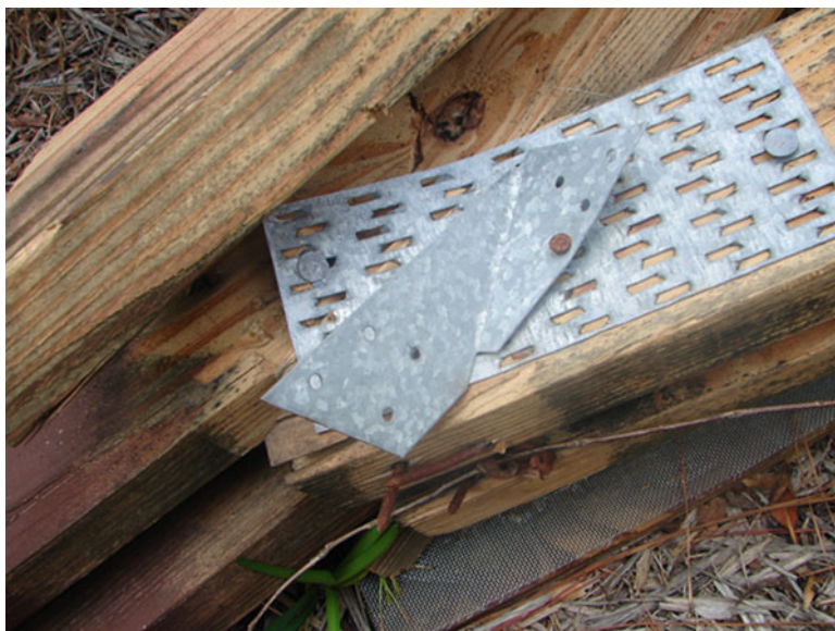
Fig. 14.10 Photo of missing fasteners in a hurricane clip. The roof lifted off after several hours of uplift pressures
