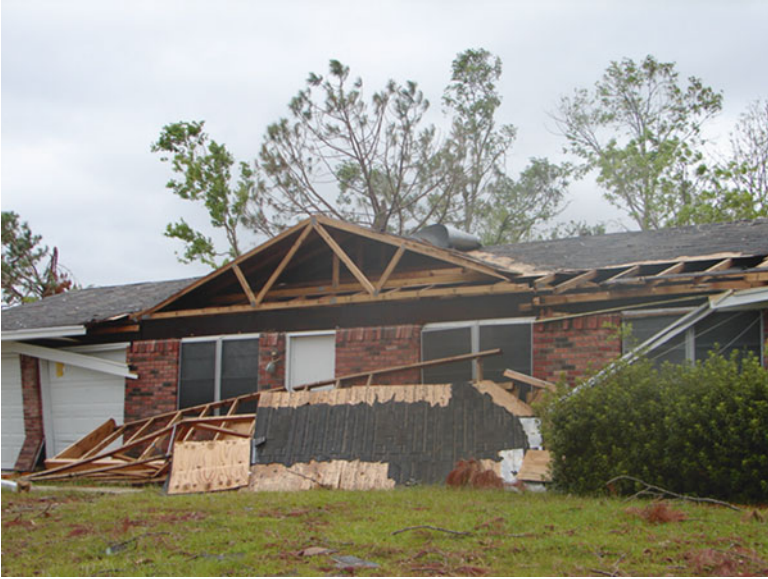
Fig. 14.7 Loss of a porch overhang due to lack of support post anchorage
