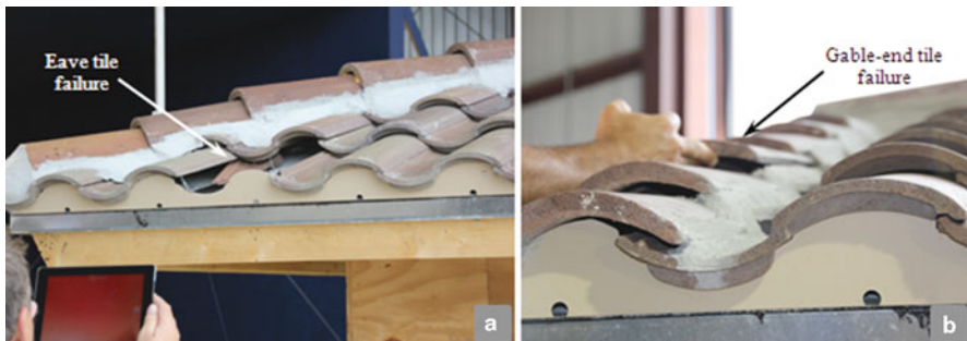
Fig. 17.9 Failure of tiles during high wind speed test. (a) Eave tile. (b) Gable-end tile (Baheru et al. 2014a)
