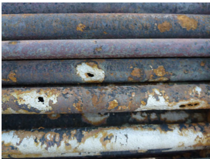
Fig. 9 Zone tube bundle corrosion damage (Zone 3)
