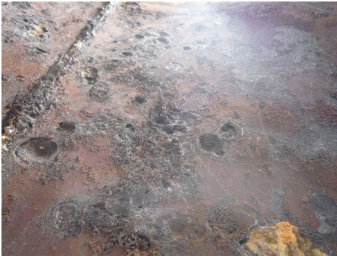
Fig. 7 Defects found in the area of AE activity corresponding to Zone 1: pitting corrosion inner surface of the heat exchanger shell
