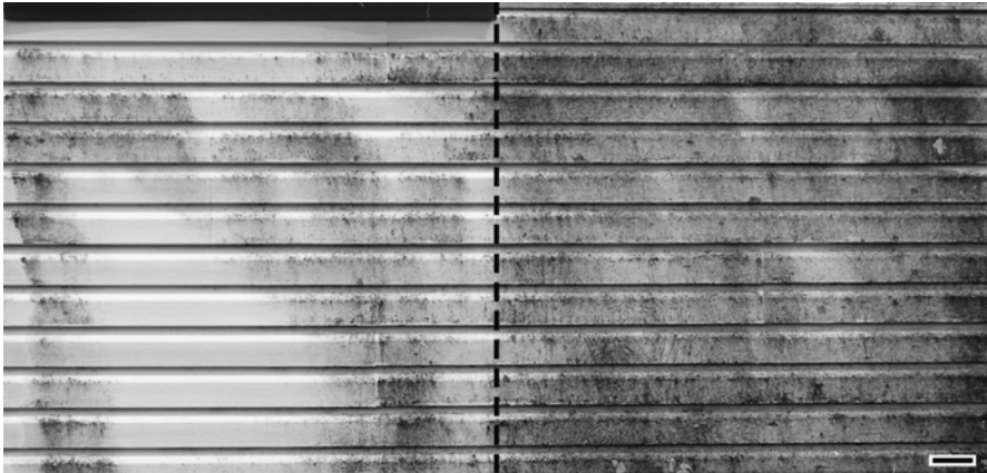
Fig. 16.3 Exterior wall panel finished in white vinyl siding. The portion of panel to the left is situated beneath a cap of metallic copper flashing, whereas copper flashing is absent at the top of the panel section at right. The area of siding located in the drainage plan beneath the copper flashing shows substantially less colonization of Baudoinia compniacensis than the unflushed portion. This is consistent with the observation of Watson et al. (1984) and their suggestion that copper and zinc may have antimicrobial potential in the management of warehouse staining (Bar = 10 cm)
