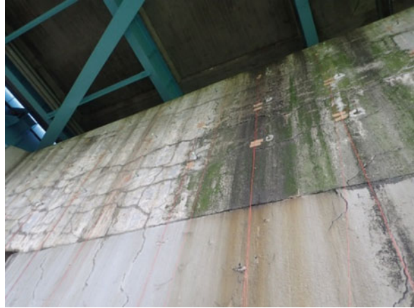
Fig. 1 Condition of surface cracks of bridge pier and sensor-attached situation (left)
