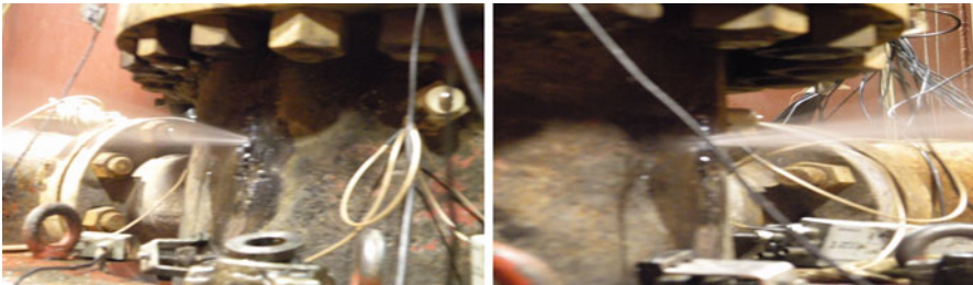
Fig. 10 The appearance when BOP shell is leaking
