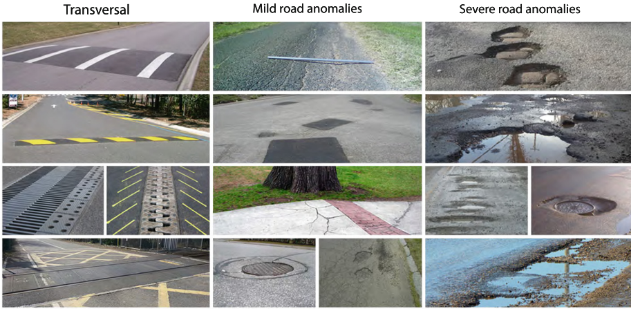
Fig. 3. Types of road anomalies
