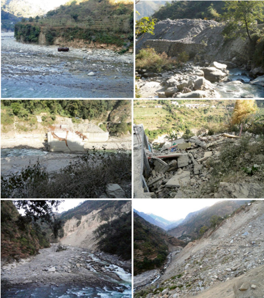
Fig. 12.6 Toe cutting by the river that destroyed the dam site (Source: Author)
