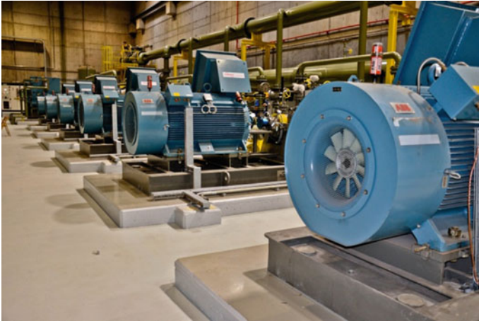
Fig. 11 Pumping station (Gorona del Viento, with permission)
