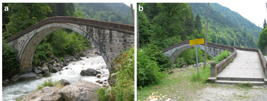
Fig. 18.6 (a, b) Historical bridges in the Firtına valley in the district Rize
