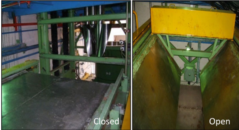
Fig. 14 Spill tray collection system
