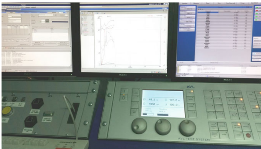
Fig. 5 Control room panels (puma open)
