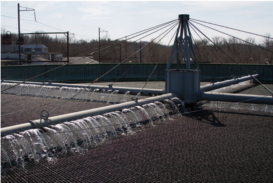
Fig. 6.2 A modern tertiary nitrifying trickling filter in operation, constructed with high-performance structured sheet PVC Media and a rotary distributor arm system (Courtesy of Brentwood Industries, Inc.)
