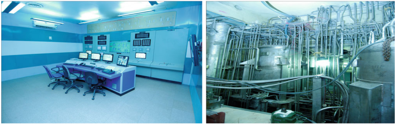
Fig. 3 Control room and in-cell extraction facility of PRTRF
