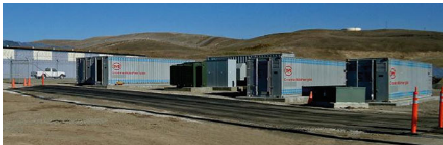
Fig. 17.6 A 2 MW Li-ion energy storage system (DOE/EPRI 2013)
