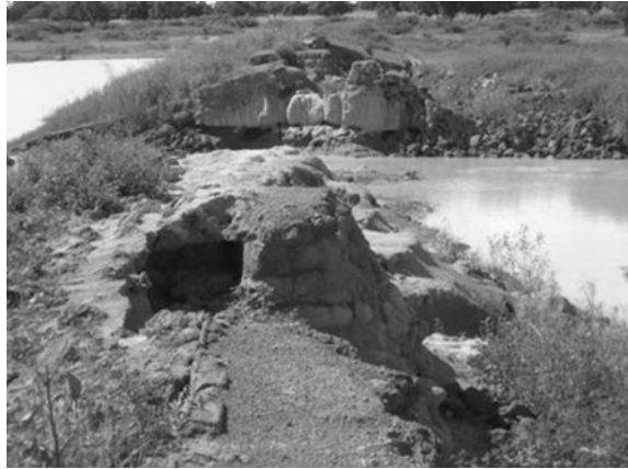
Fig. 4.3 Collapsed dyke at Tanghin. Photo by authors
