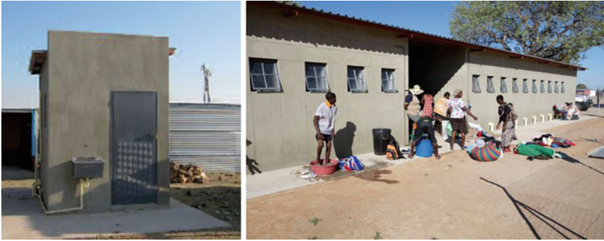
Fig. 26.11 A cluster washhouse ( left ) in Tobias Hainyeko settlement and the communal washhouse ( right ) in Okayekongwe settlement of Outapi
