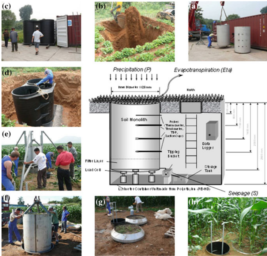
Fig. 20.3 Construction of the lysimeter facility at the Shixia research station: a prefabricated lysimeter station after the seaway transport; b pit for the lysimeter station; c preparation of the steel lysimeter vessels; d insertion of the prefabricated lysimeter container station; e monolithical extraction of the lysimeter soil column; f insertion of the lysimeter vessel into the container lysimeter station; g view to the almost finished lysimeter station with two lysimeter vessels and a manhole for inspection and maintenance; h maize plants at the finished lysimeter station in July 2011; i principal sketch of the weighable container lysimeter station
