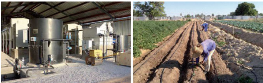
Fig. 26.12 View into the main building of the wastewater treatment plant and on the irrigation site for agricultural production under reusing water and nutrients
