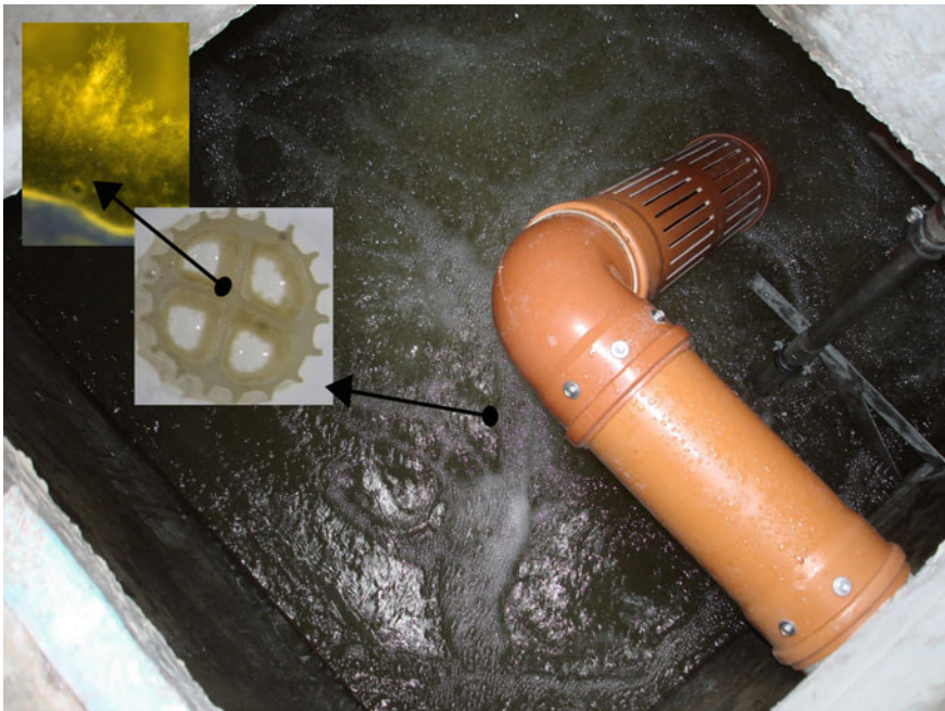
Fig. 25.12 Biological stage with plastic carrier media and biofilm. Source Bergmann Beton + Abwassertechnik GmbH
