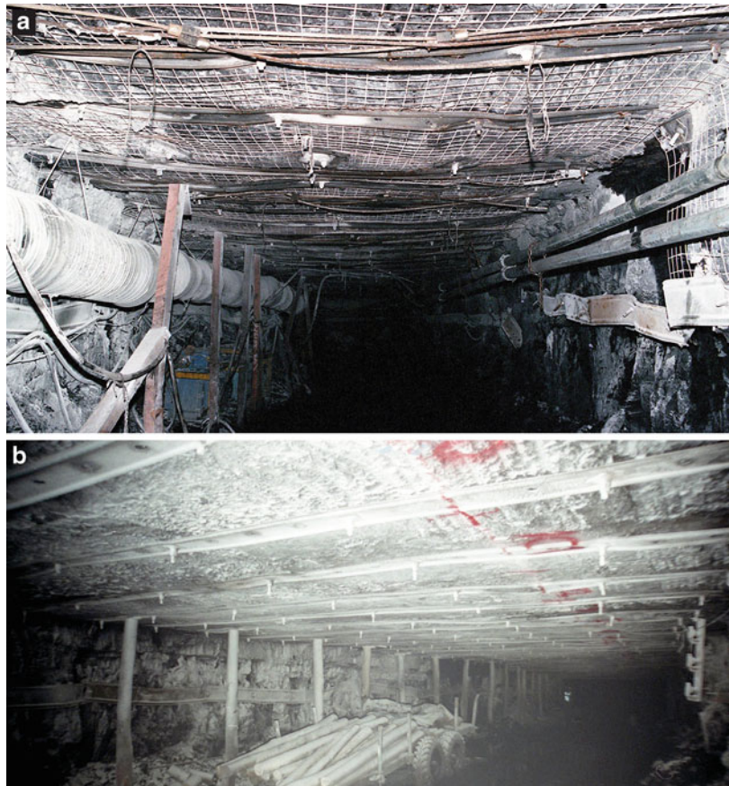
Fig. 9.24 An example of the beneficial effect on ground control of utilising a sacrificial roadway to create a lateral stress shadow in a high horizontal stress environment. (a) A 4.8 m wide cut-through driven at \sim 65^\circ to the regional major horizontal stress, which was \sigma_1 (b) An 8 m wide longwall installation roadway driven from the cut-through shown in (a) after the formation of a 10 m wide caved sacrificial roadway some 9 m further inbye
