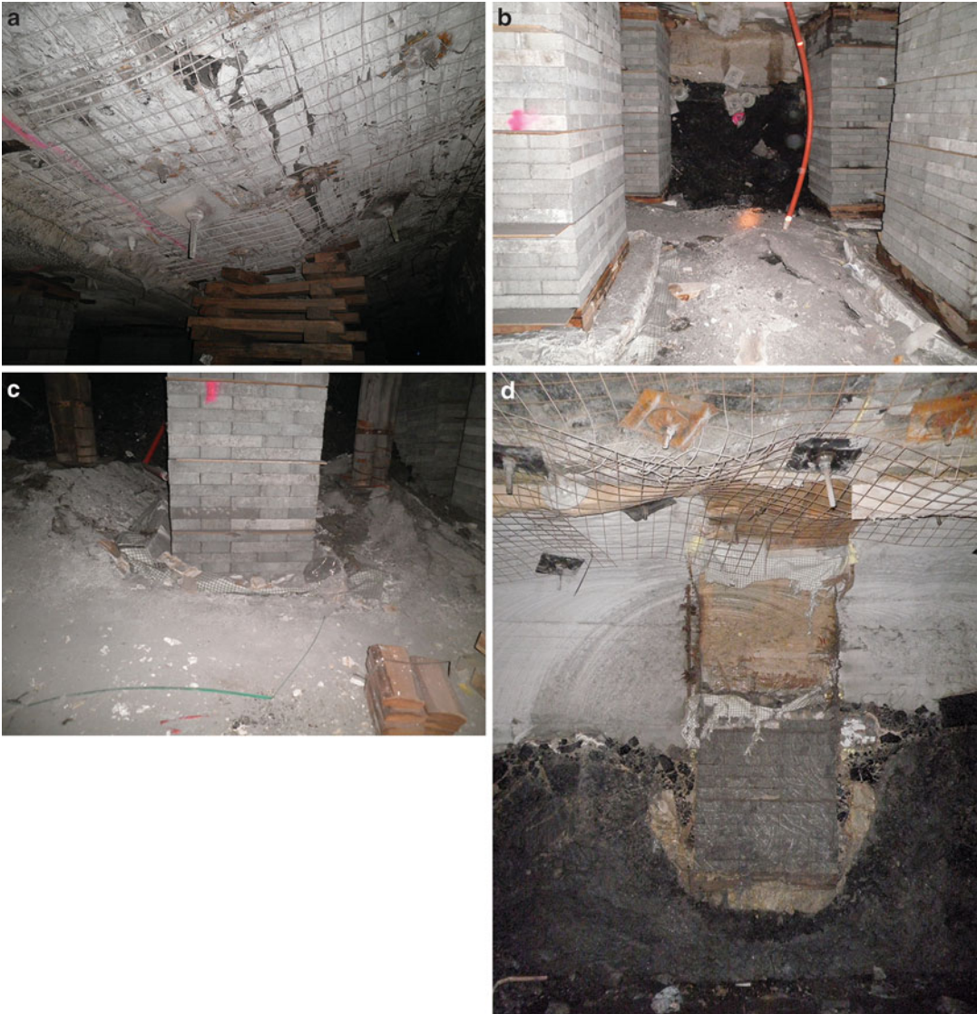
Fig. 9.26 Failure of a pre-developed roadway in 2011 at an Australian colliery, associated with punching of fender and standing supports into soft and weak floor under deadweight load of a detached block. (a) Pivot point of
