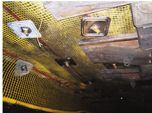
Fig. 9.28 A longwall recovery roadway that has been supported with polyester screen and bolts
