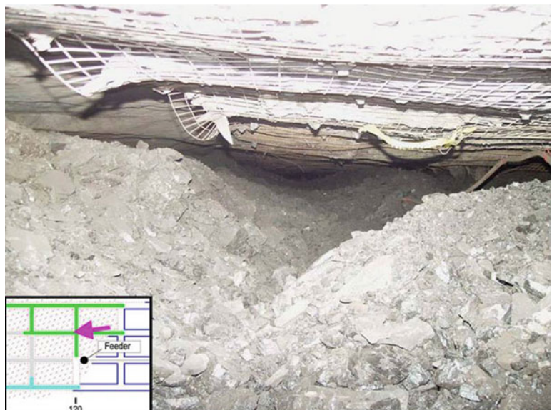
Fig. 4.32 View of No. 3 entry after 7 August 2007 burst at Crandall Canyon Mine (After Gates et al. 2008)
