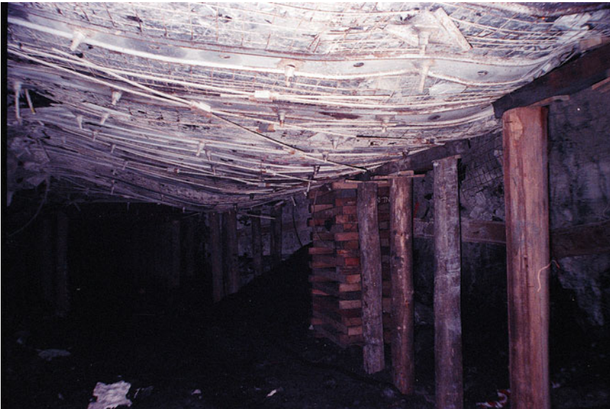
Fig. 6.33 An example of failed immediate roof suspended off the excavation abutments by means of long tendons angled over the ribline and trussed across the excavation
