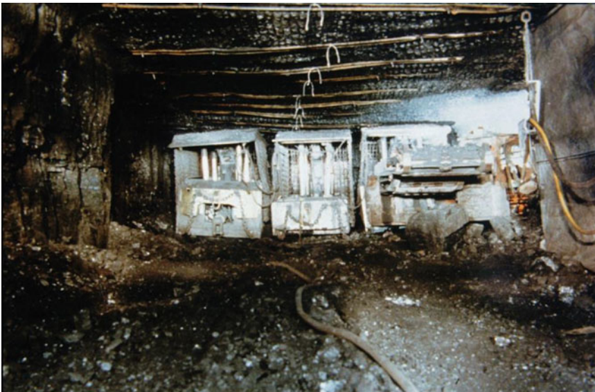
Fig. 8.14 Lifting left and right using three MRS at an Australian colliery – right hand MRS partially obscured by the tail boom of the continuous miner
