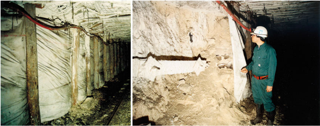
Fig. 7.7 An example of rib replacement to mitigate the effects of severe rib spall of the type shown in Table 7.8e (After Galvin 1996).
