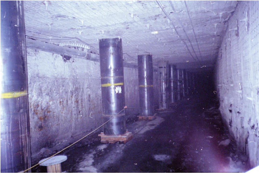
Fig. 6.12 700 mm diameter CAN ® proprietary brand monolithic cementitious chocks installed in a longwall tailgate
