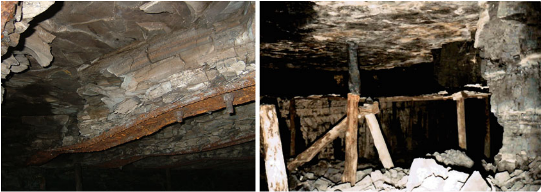
Fig. 6.55 Examples of the types of roof conditions that can benefit from support systems that incorporate screens
