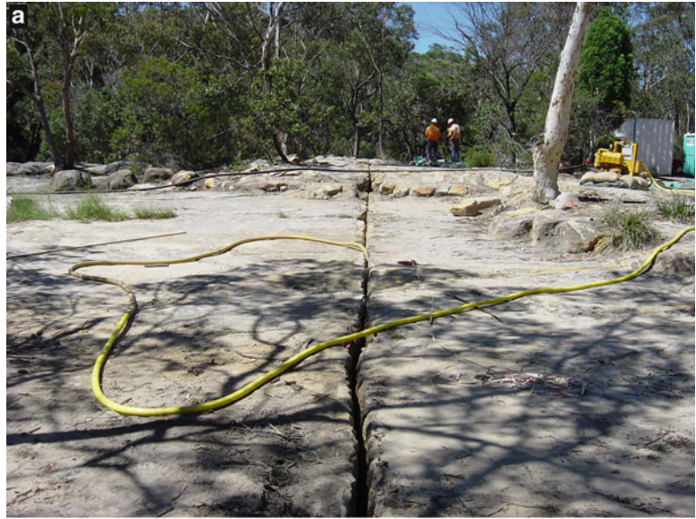
Fig. 10.34 Illustration of the use of a slot to mitigate subsidence impacts on a rock bar at Marhnyes Hole on the Georges River in the Southern Coalfield of NSW, Australia. (a) A slot created adjacent to a river rock bar by drilling series of closely spaced boreholes in order to mitigate subsidence-induced movements at the rock bar. (b) Differential displacement across the slot shown in (a) , demonstrating the level of protection from strain provided to the rock bar
