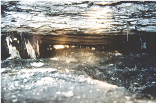
Fig. A4.3 Bearing capacity failure beneath abutment pillars in partial pillar extraction workings, resulting in some 2 m of closure in 2.7 m high workings
