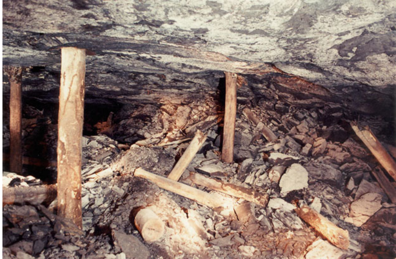
Fig. 4.31 A pillar that is in the process of failing in a controlled manner
