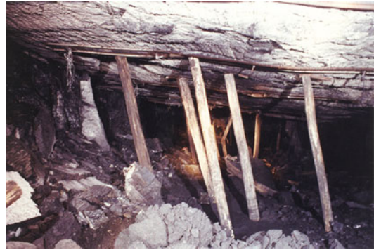
Fig. A4.4 Extrusion of foundation material from beneath a pillar as evidenced by the angle of the props and the condition of the pillar side
