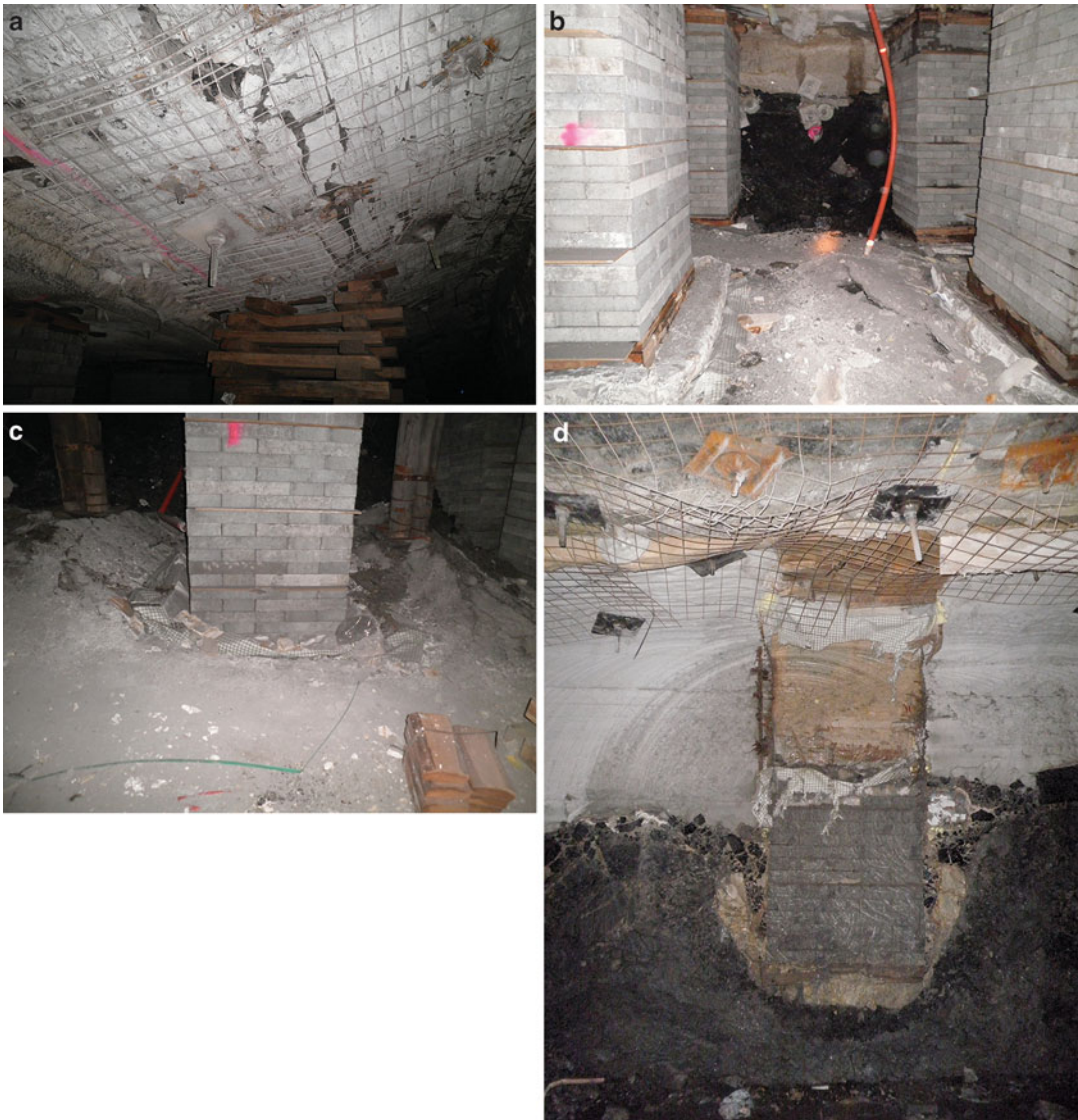
Fig. 9.26 Failure of a pre-developed roadway in 2011 at an Australian colliery, associated with punching of fender and standing supports into soft and weak floor under deadweight load of a detached block. (a) Pivot point of
