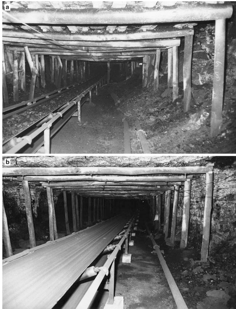
Fig. 6.15 Change in roof and rib conditions in the Greta Seam, Australia, brought about by the introduction of rock bolting. (a) Roof and rib conditions preceding the introduction of roof bolting, (b) Roof and rib conditions following the introduction of roof bolting – alternative rows of timber supports reflect mine workers initial concerns about the effectiveness of roof bolts and W straps
