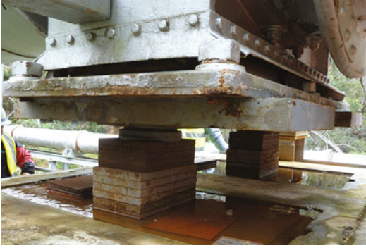
Fig. 10.36 Jacking and packing of a riveted wrought iron aqueduct spanning a valley to compensate for upsidence during undermining by a longwall panel
