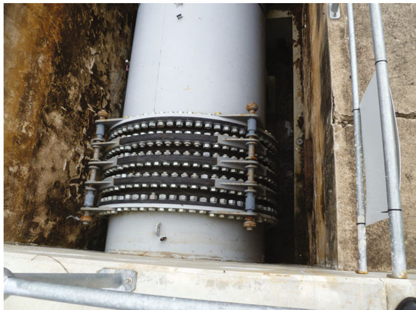
Fig. 10.35 Rubber bellows to mitigate against valley closure, retrofitted into the abutment end of a 2.44 m diameter wrought iron aqueduct spanning a valley
