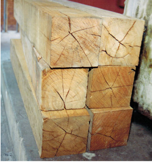
Fig. 6.8 Chock timber elements adversely affected by having been cut from heartwood (After Galvin et al. 1996)
