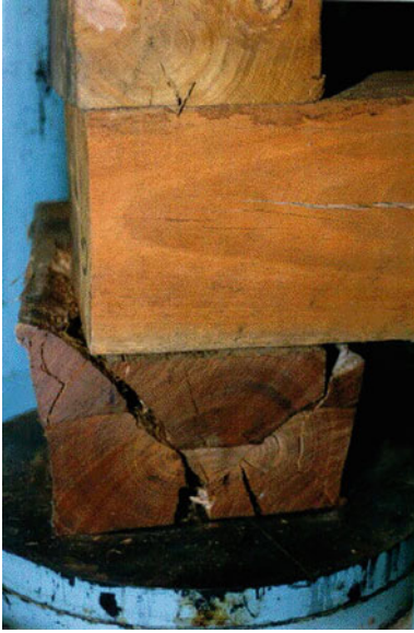
Fig. 6.11 Shear failure of the end of a chock timber due to insufficient overhang between timber layers (After Offner et al. 1999)
