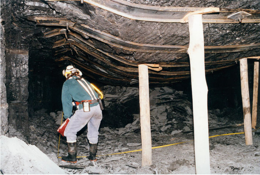
Fig. 6.32 An illustration of the effectiveness of angled bolts installed towards the abutment in controlling failure of a laminated coal roof
