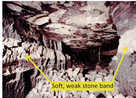
Fig. 4.15 Rib spall caused by the extrusion of a soft and weak stone band within the extraction horizon
