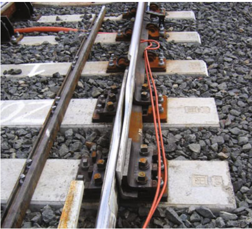
Fig. 10.37 Tapered switchblades and real time monitoring installed in the main Sydney to Melbourne railway line (Australia) above an active longwall panel in order to manage mining-induced strain in the rails (After Pidgeon et al. 2011)
