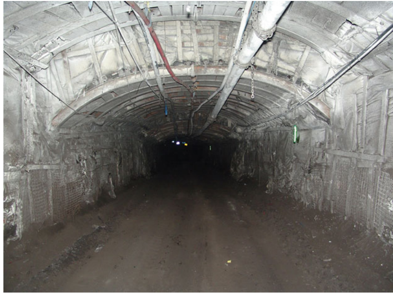
Fig. 6.14 Steel arches, lagging and rib replacement used to support a severely disturbed geologically zone
