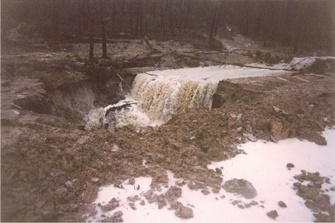
Fig. 3.32 An example of a watercourse breaking through into shallow pillar extraction workings during a rainfall event
