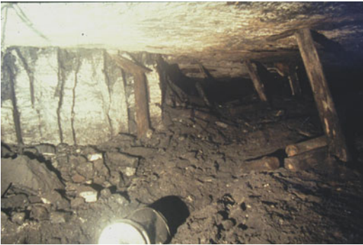
Fig. 4.19 Extrusion of weak floor material from under a pillar, causing open vertical cracks to develop through the full width of the pillar under the influence of induced lateral tension
