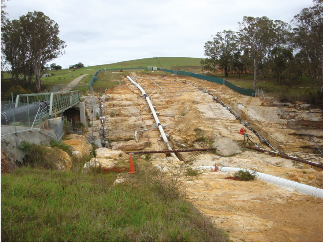
Fig. 10.33 Decoupling of pressurised gas pipelines and water mains from mine subsidence-induced ground movements, in particular valley closure and upsidence
