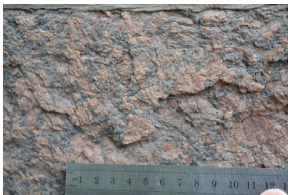
Fig. 2 Exfoliation of granite (St. Petersburg, Facade of Russian museum building)
