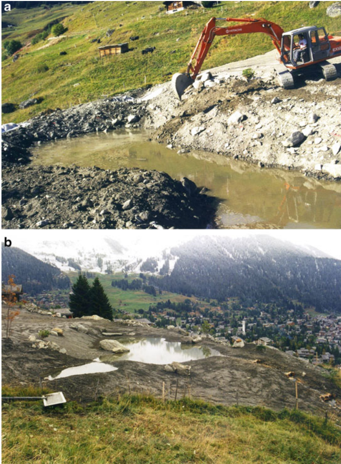
Fig. 3.13 Pond dug in the Swiss Alps (1800 m.a.s.l.). The technical difficulties are often linked to the topography, with machinery having to navigate steep slopes (photos: P.A. Frossard)
