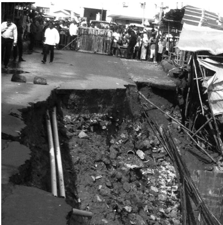
Fig. 10.2 Sierra Leone’s collapsed King Jimmy bridge along Wallace Johnson Street in Freetown, August 2013
