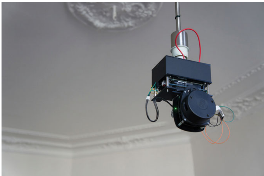
Fig. 20 Scanner installed to the lamp socket for 3D scanning of the room
