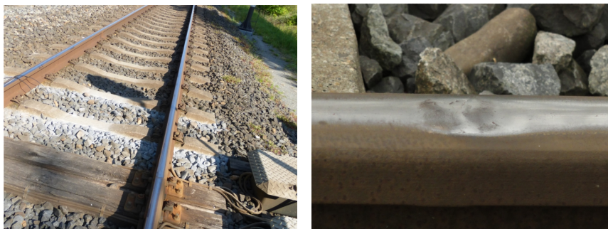
(a) Loose ballast indicated by the presence of white dust
