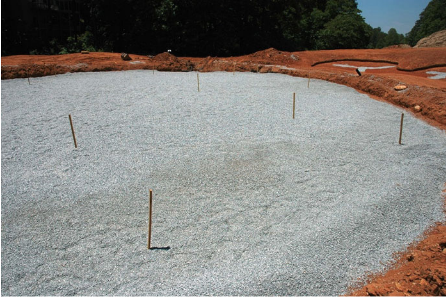
Fig. 2.32 Grade stakes to clearly mark proper depths of various components of layered systems
