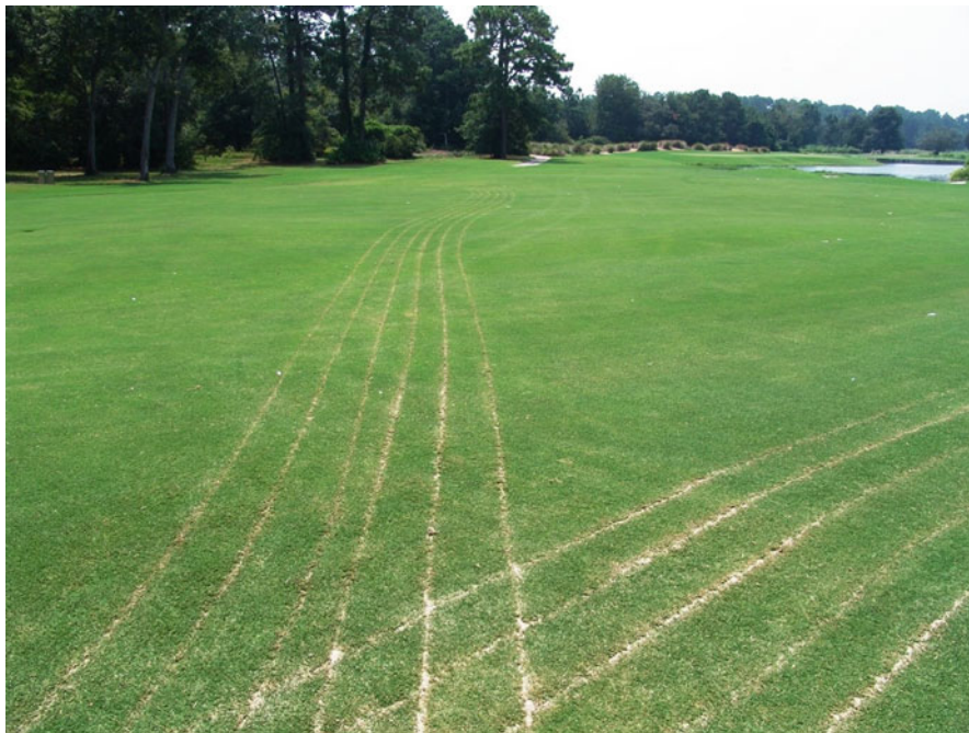
Fig. 2.24 Narrow slit drains backfilled with sand to reduce surface moisture. This helps lower the water table until the slits fill with water
