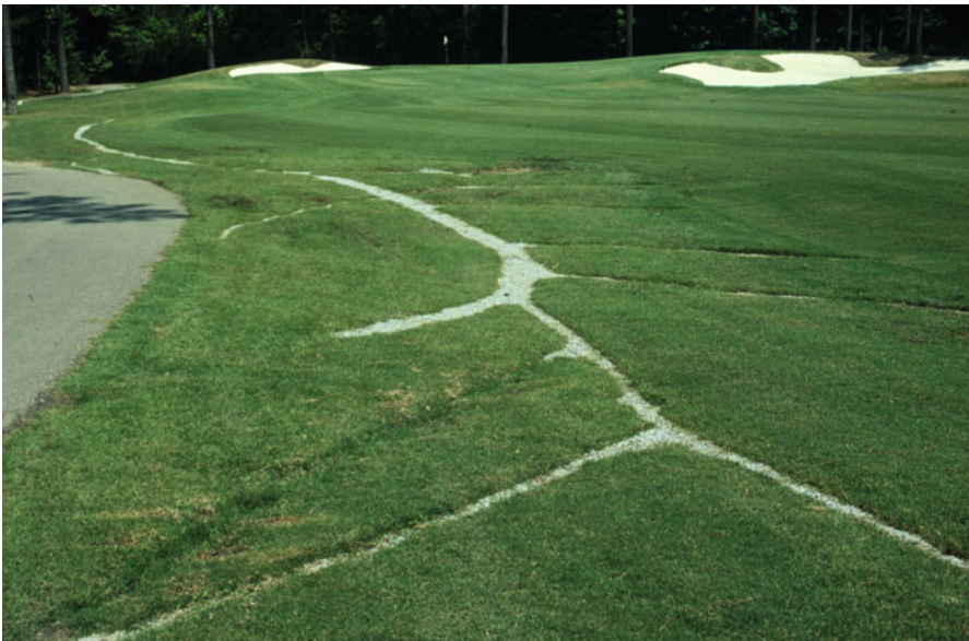
Fig. 2.22 Installation of slit drains (also called French drains) in a fairway where a 4 to 8 in (10 to 20 cm ) wide trench is backfilled with sand. A drain tile may also be placed at the bottom of these to facilitate water removal
