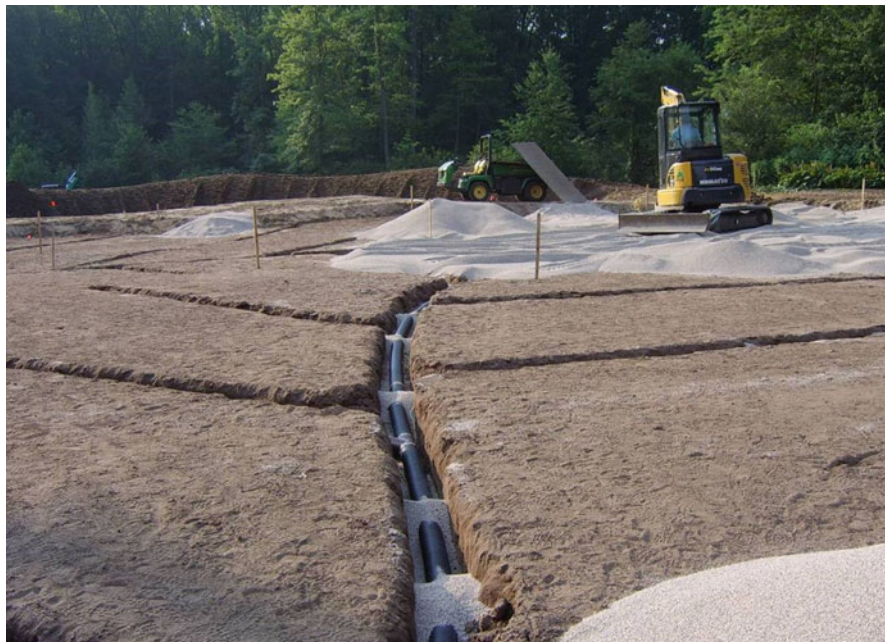
Fig. 2.26 Trenches in golf green subsoil with drainage tile and being backfilled with gravel
