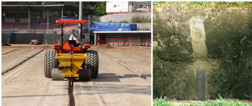
Fig. 2.50 Installing slit drains (also referred to as “cell system”) where a narrow trench is backfilled with sand to remove excess surface moisture ( left ); A 1 to 2 in diameter (2.5 to 5 cm) pipe placed at the bottom of the trench to facilitate water removal ( right )
