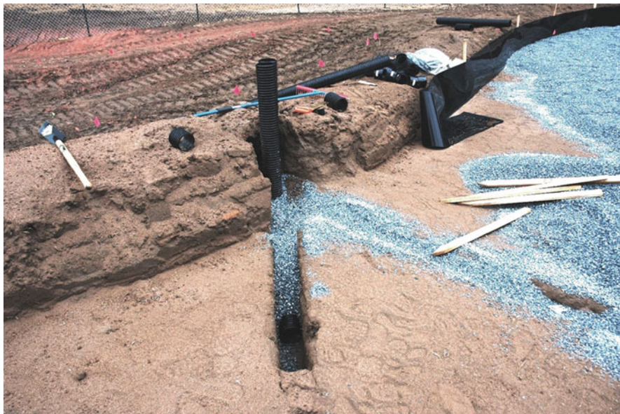
Fig. 2.33 Main tile line extended to the soil surface and capped to allow future clean-out if clogging is suspected
