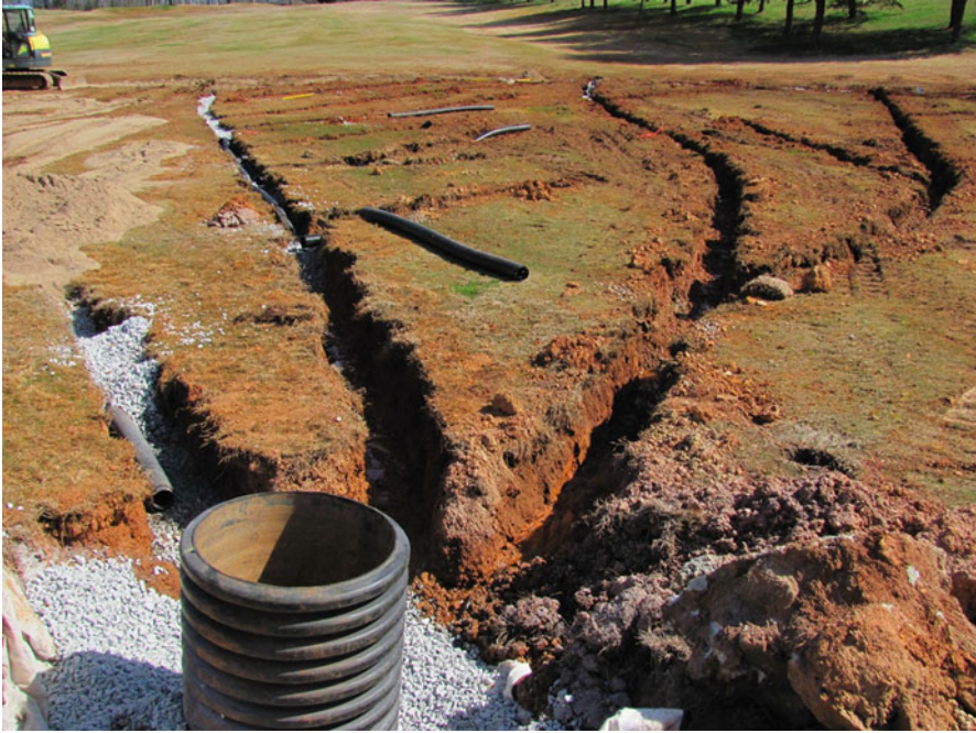
Fig. 2.38 Collection point for several main lateral drainage lines. The collected water is then removed or redistributed away from the property
