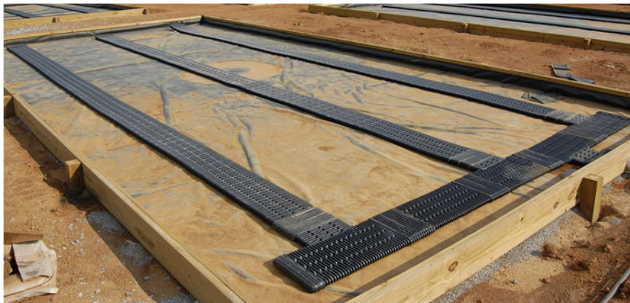
Fig. 2.31 Flat panel tile being used instead of the traditional round perforated tile. Flat panel tile is laid on the subgrade and not imbedded into it saving trenching and spoil disposal costs
