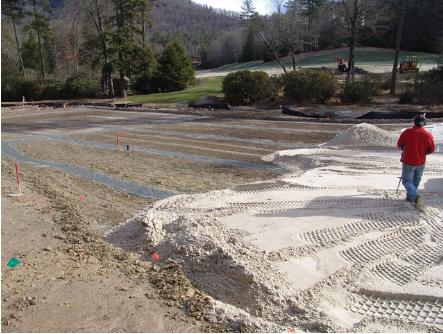
Fig. 2.39 Sand capping a perpetually wet site to raise the turf above the naturally occurring high water table
