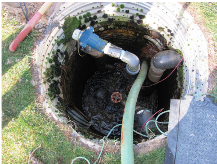
Fig. 2.29 Sump and pump to removed water from a drainage system
