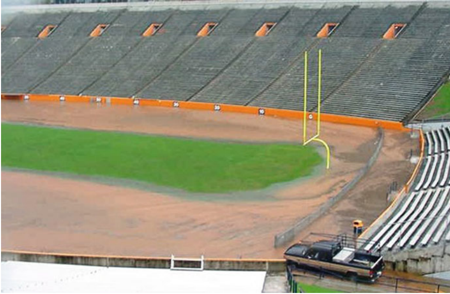
Fig. 2.11 “Bathtub” effect of inadequate surface and subsurface drainage due to underlying clayey soils without sufficient drainage and outlets for the amount of rainfall received
