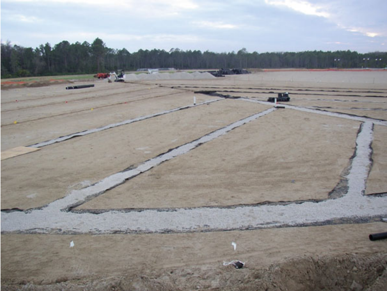
Fig. 3.13 Successful greens and sports fields have been constructed without the 4 in (10 cm) pea gravel layer. However, drainage trenches should be backfilled with gravel
