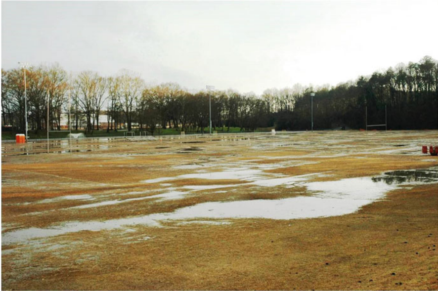
Fig. 3.23 Proper construction produces a field with good surface and subsurface drainage that is easier to maintain and quicker to resume activity following heavy rainfall. With increasing interest in playing athletic events on time to satisfy television contracts, proper drainage is a must for higher profile fields. Unamended, native soil fields (shown) often drain poorly, eventually rutting and puddling excessively
