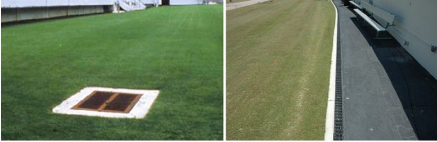
Fig. 2.45 Traditionally used surface catch basin to capture excessive surface water ( left ); strip surface drains to capture excessive surface water ( right )
