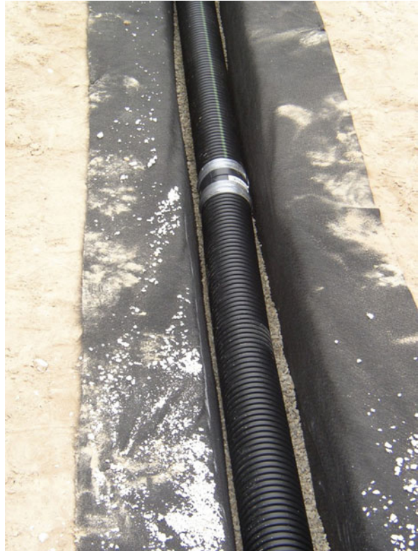
Fig. 2.15 Four inch in perforated tile placed into the subgrade and back-filled with gravel to help facilitate subsurface drainage
