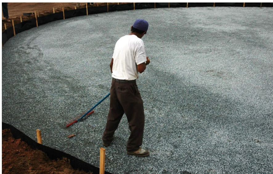
Fig. 3.12 In golf green and sports field construction, after the drains are installed, the packed subgrade can be covered with 4 in (10 cm) of “pea” (1/4 to 3/8 in diameter, 6.4–9.5 mm) gravel conforming to the proposed final surface grade of the green to a tolerance of \pm 1 in (2.5 cm)
