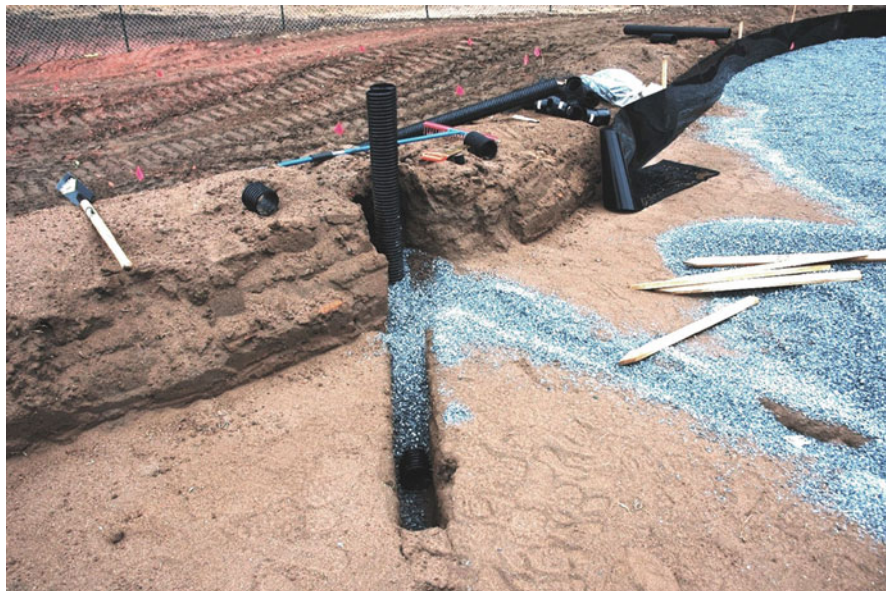
Fig. 2.33 Main tile line extended to the soil surface and capped to allow future clean-out if clogging is suspected
