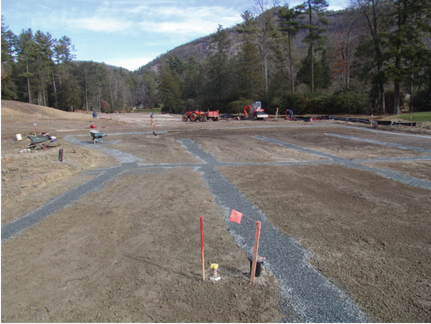
Fig. 2.34 Subsurface drainage being installed on a golf course fairway. Drainage ditches are back-filled with gravel prior to soil placement
