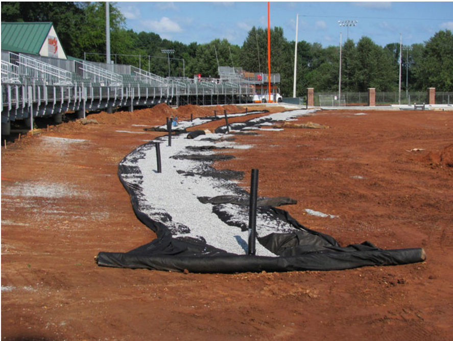
Fig. 2.55 Installing a perimeter drainage line adjacent to the warning track of a baseball field
