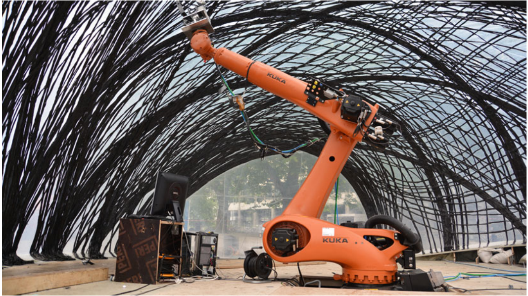
Fig. 4 Experimental fabrication set up of primary and secondary fibre bundles on pneumatic formwork
