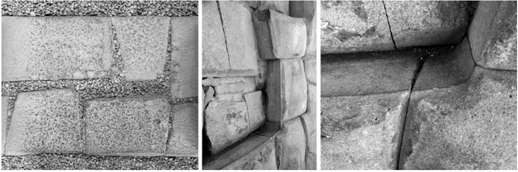
Fig. 3 A series of Inca constructions that reveal the voided wedge between stones
