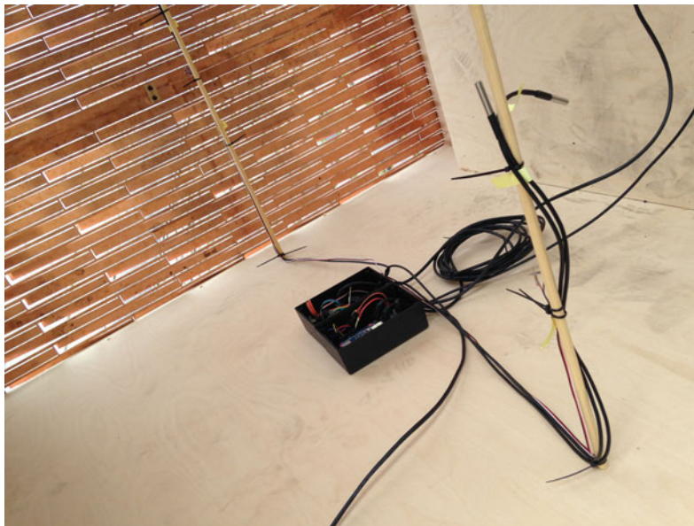
Fig. 4 Sensors and microprocessor installed for post-construct analysis just inside the membrane and in the back of the space. The prototype consists of 24 panels with the dimensions 490 \times 1490 mm. Six clusters of four
