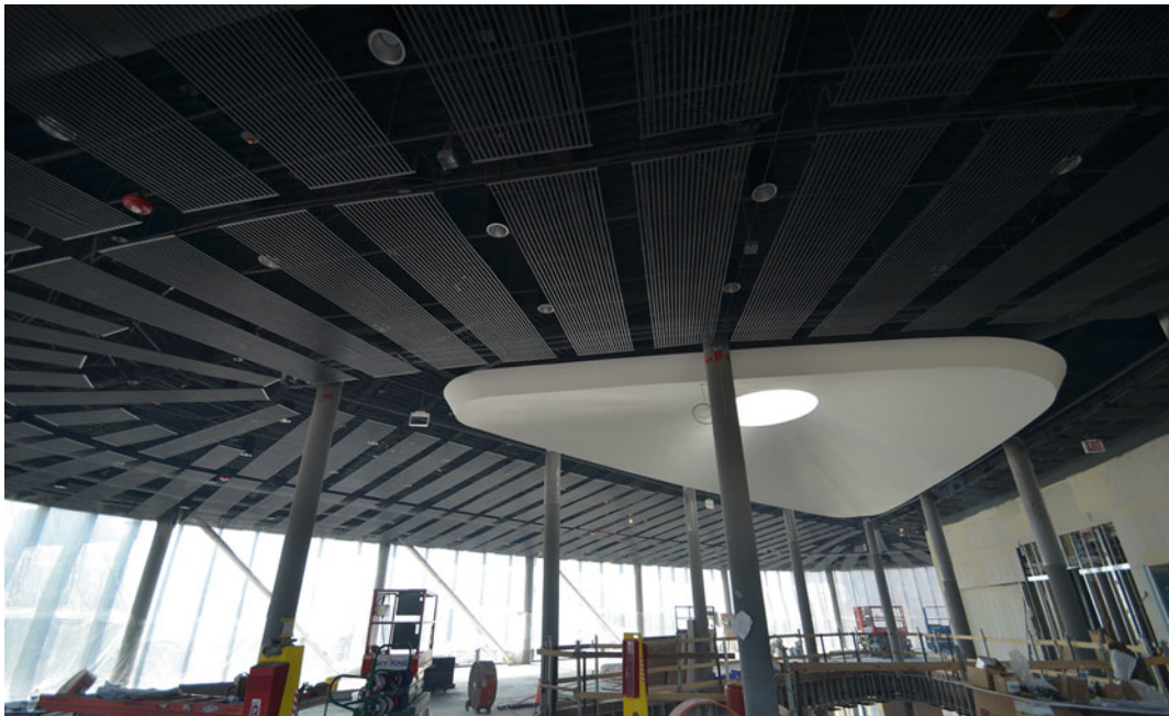
Fig. 2 Construction photo of Chicago Chinatown branch library and capillary radiant mat installation
