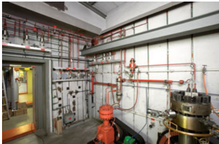
1000-bar compressor room
