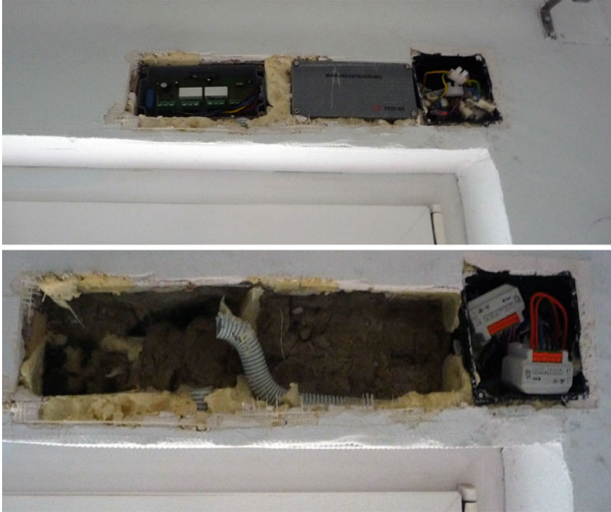
Fig. 7.8 The figure shows the changes in component size between the first installation on the top and the second version on the bottom
