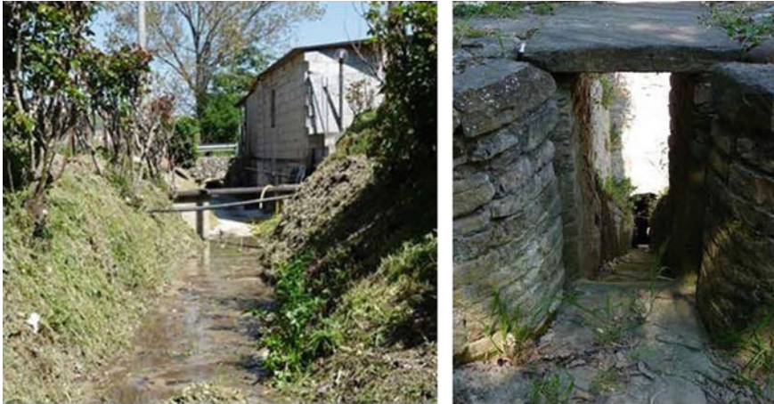
Fig. 6 Soil diversion channel photos. On the right , the last stretch of the channel, just upstream of the mill
