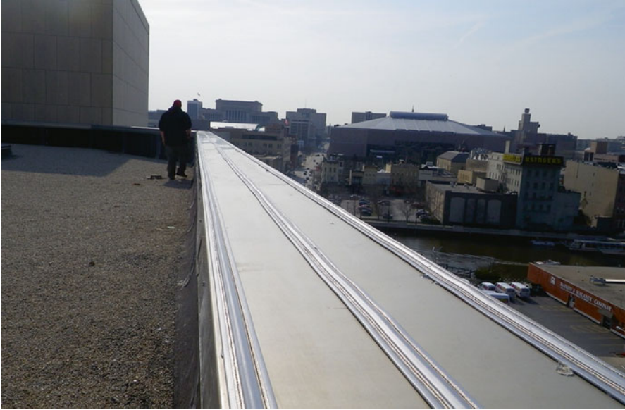
Fig. 9.4 Electric shock track used to keep birds off of the building's ledge. Photo by Carla Wagner
