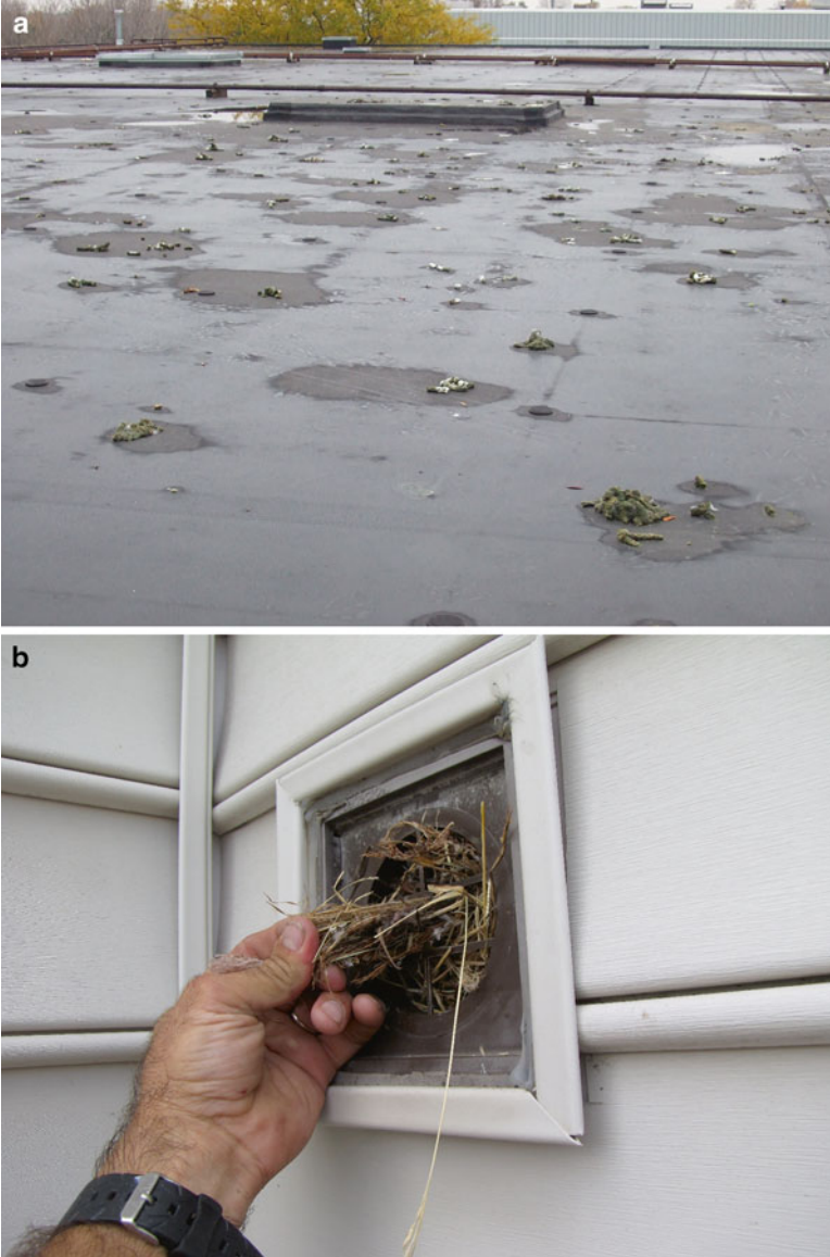
Fig. 9.1 (a) Feces of Canada geese on a roof can clog drains and lead to roof collapse from the weight of accumulated rain water. Photo by Carla Wagner. (b) Starling ( Sturnus vulgaris ) nest has plugged this dryer vent which could have caused a fire. Photo by Kevin Cornwell
