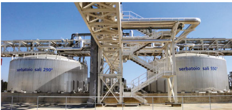
Fig. 3 Heat storage system installed in the Archimede plant
