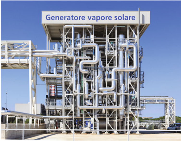
Fig. 4 Steam generator of the Archimede plant
