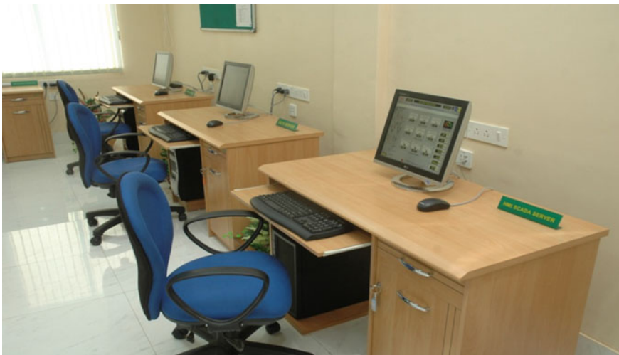
Fig. 7 SCADA room at Mongol Pandey water treatment plant
