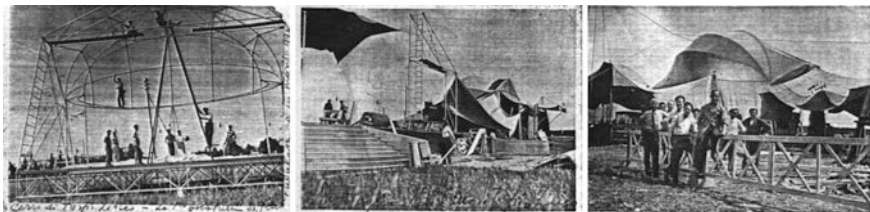
Fig. 1.6 Assembling phases of the dome of a Tespi lyric theatre, by the Italian Workshop of Waterproof Fabrics, 1928 (Source Cardone and Coccu 2005)
