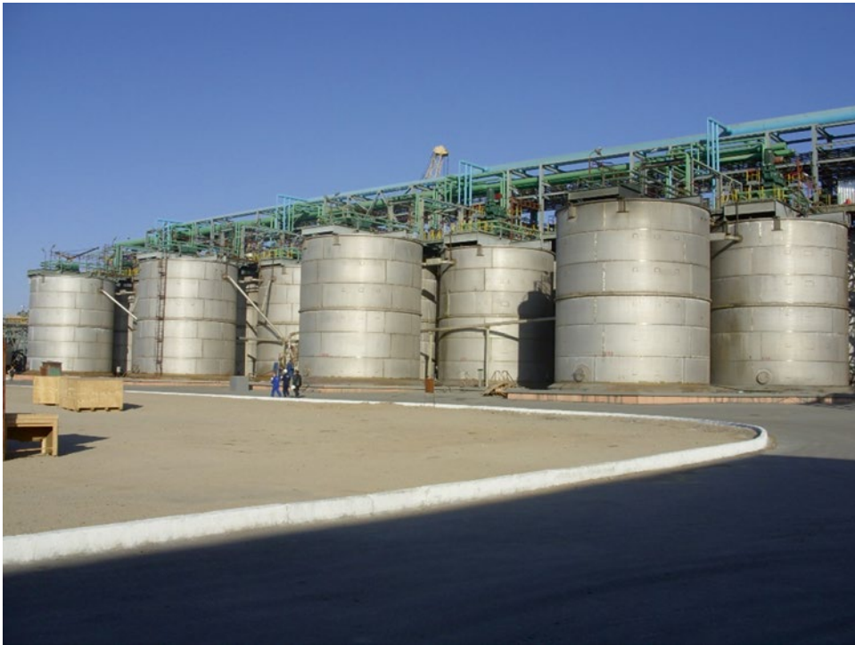
Fig. 6.3 CSTR biooxidation circuit at the Kokpatas, Uzbekistan BIOX ® plant (photo courtesy of Biomin South Africa (Pty) Ltd.)
