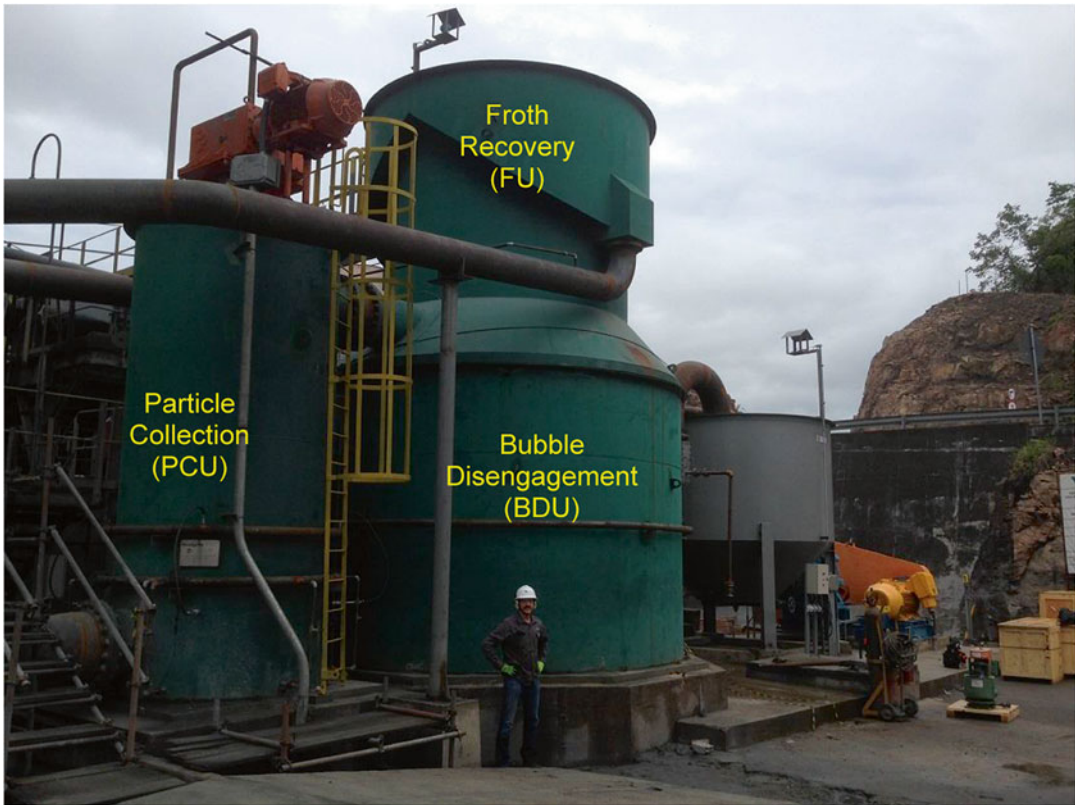
Fig. 2.12 Installation of staged flotation reactor (SFR) in an operation (with permission from Woodgrove technologies)
